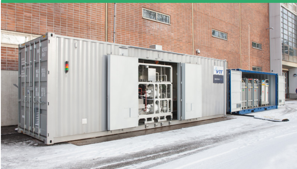
Figure 14. Containerised pilot unit for the production of hydrocarbons from carbon dioxide and hydrogen.
