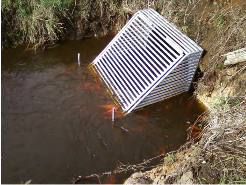
Figure 2. Permanent fish barrier installed on downstream side of road culvert outlet to Lake Ohinewai showing around 60 adult koi carp attempting to pass the barrier.
