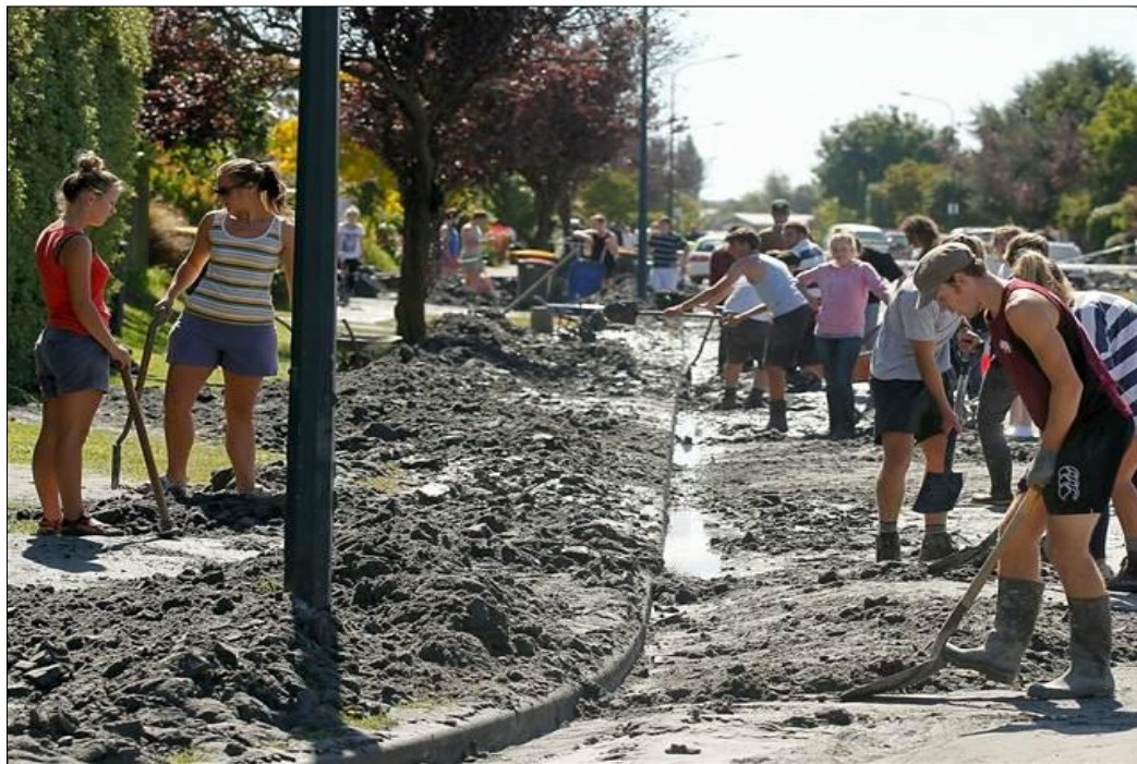
Figure 2.4: Student Volunteer Army (SVA) removing mud and silt from east Christchurch Source: Platt (2012: 34)
