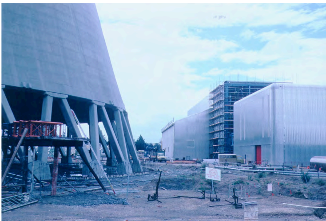
The cooling tower and power station, Ohaaki, May 1987
