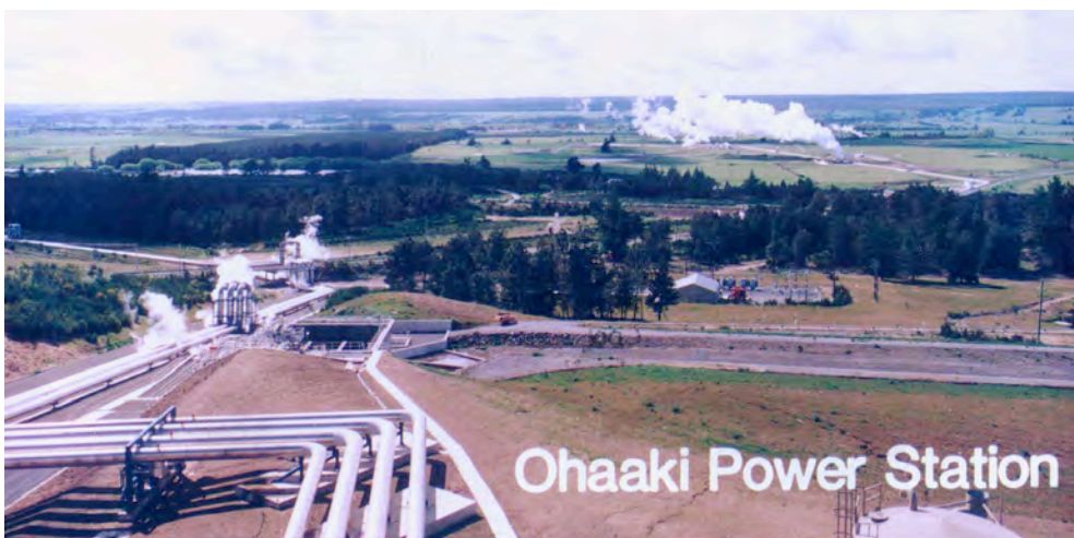
Views of Ohaaki power project site from the power house looking across Reporoa Valley to the Kaingaroa Forest: top construction work, May 1984; middle , view from the power house, 1986; bottom , the completed steam field pipework in 1989 (Electricorp photo).
