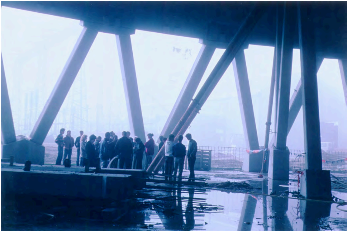
Inside the cooling tower on a winter day in June 1987: looking up to the blue sky above and standing in the Reporoa fog below.
