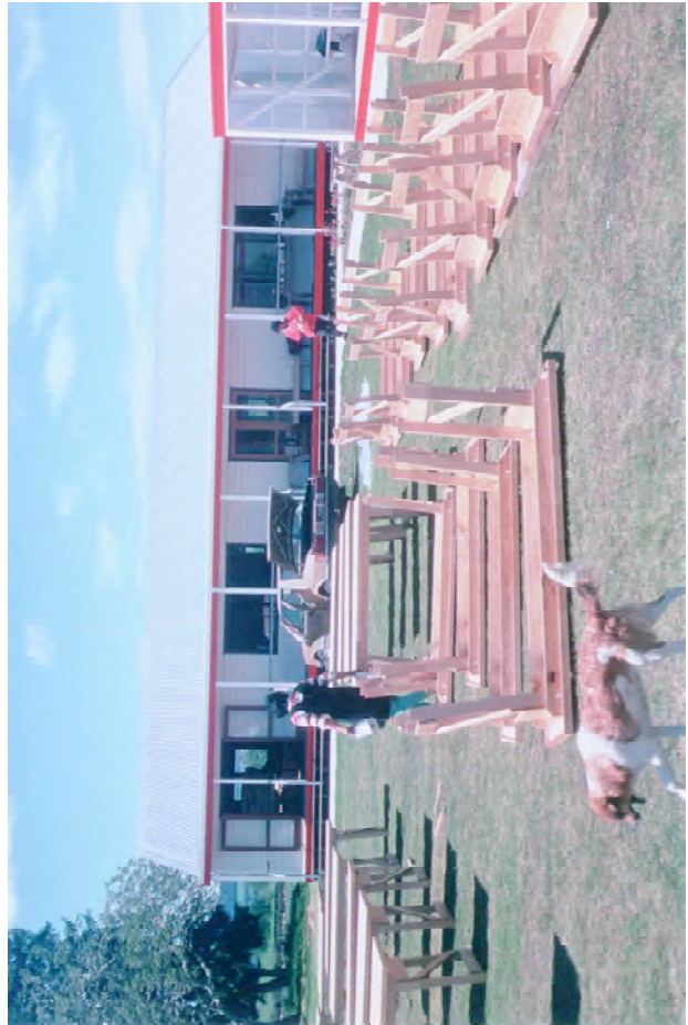
The new dining hall, Wairakewa, at Te Ohaaki Marae in 1989; top left , construction of shelter for marae speakers; bottom left , varnishing the furniture; right , putting the finishing touches on a new flagpole.
