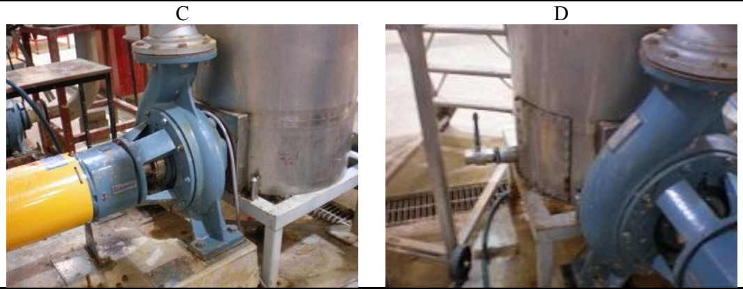
Figure 13: Comminution system. A – 600 L stainless steel tank. B – Tank filled with 300 L water. C – Scanpump connected to side of tank. D – Side access panel and discharge valve.
