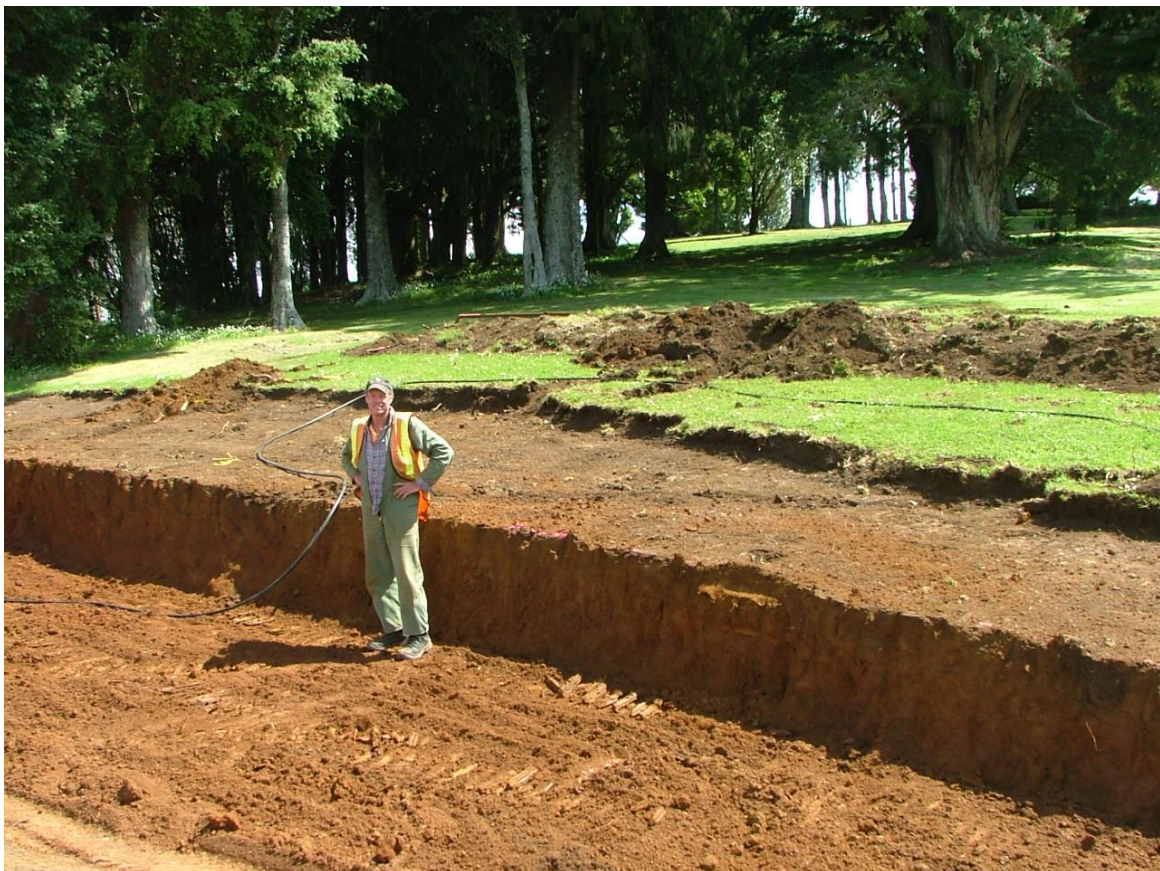
Freshly exposed Pukekohe soil at top of Anzac Rd, Pukekohe Hill, on 10 October, 2008. Leo provides the scale for new road turn-around under construction. Photo: David Lowe
