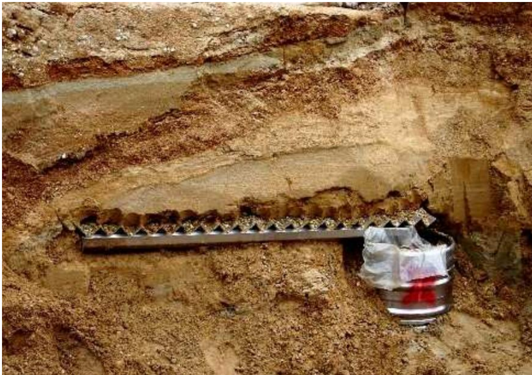
Figure 2.3: A zero-tension gravity pan lysimeter during installation. Note undisturbed soil above the pan (from Peters & Durner, 2009).
