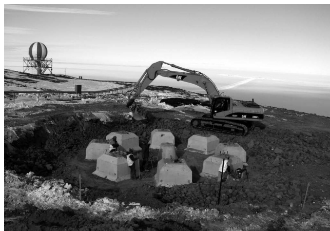
Foundations going in for the proposed windfarm site on Ross Island, Antarctica. (Photograph provided by Megan Balks)
