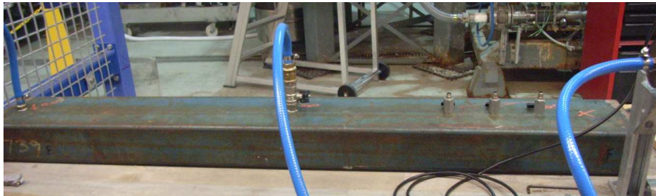
Figure 4.4, Manifold with inlet from supply and various outlets.
