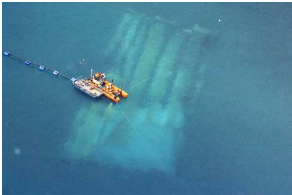
Figure 1.3. Aerial photographs of the site during reef construction. The reef is made of sand-filled geotextile containers and is located about 250 m from the shore. (Source: Mount Reef website: www.mountreef.co.nz ).
