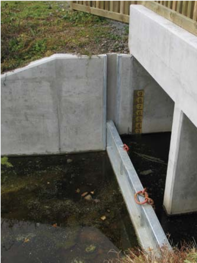
Culvert with removable concrete inserts to enable further hydrological manipulation when required. Photo: Wildland Consultants Ltd.
