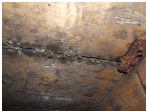
Figure 3.8: Photograph of actively growing mould under the kitchen table in the galley area at Terra Nova Hut (2004).
