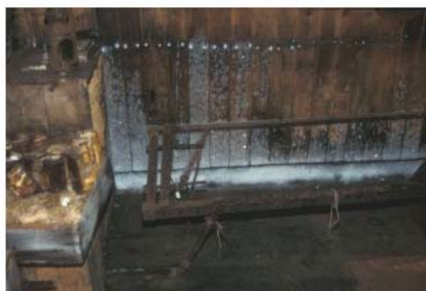
Fig. 4. Frost accumulation inside Cape Evans hut at the base of the south wall in the galley. When temperatures rise above 0°C the frost melts producing sufficient moisture for mold growth in this area.
