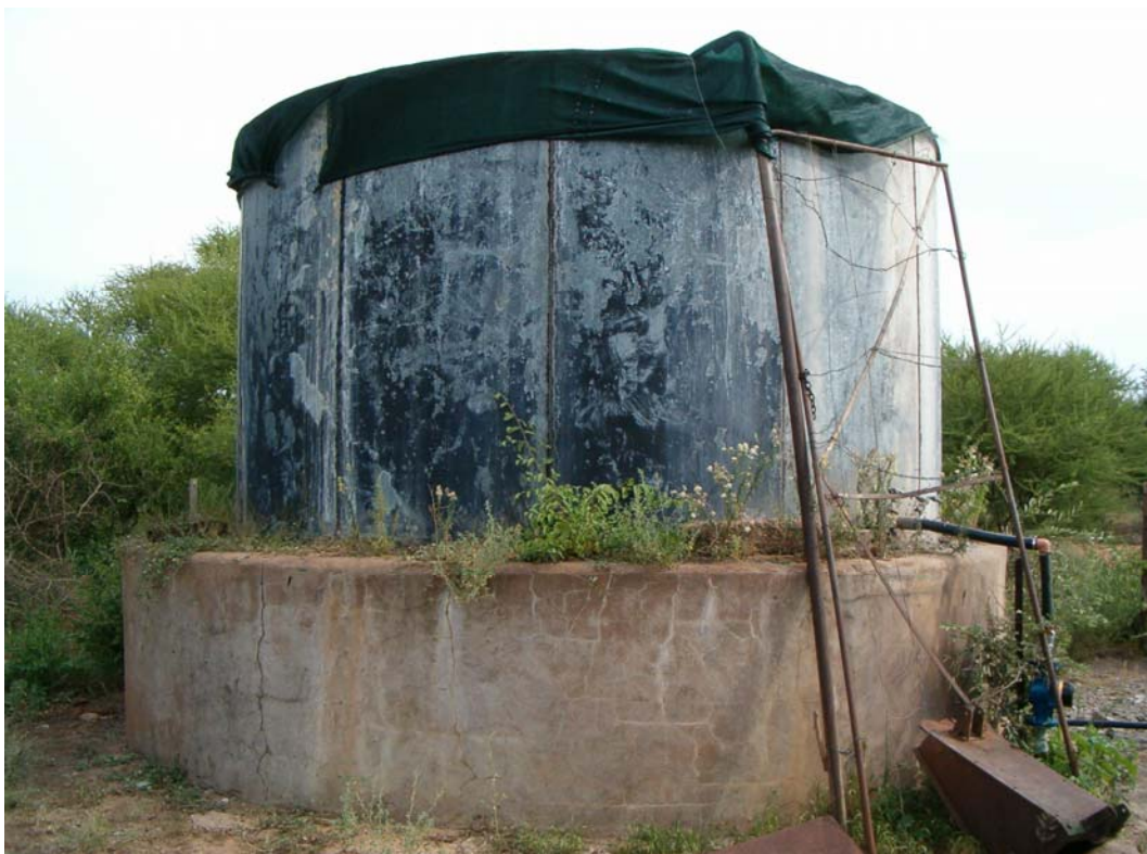
Figure 8.2: Water storage tank in Masama Ranch.
