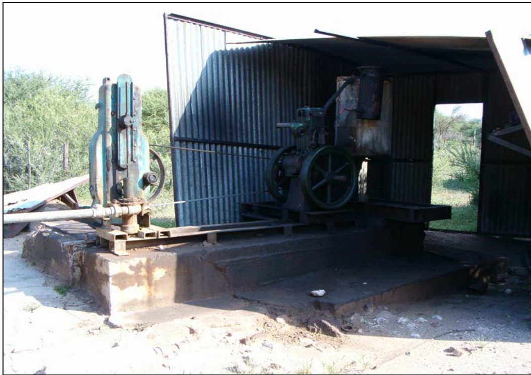
Figure 8.1: Borehole and pump in Masama Ranch
