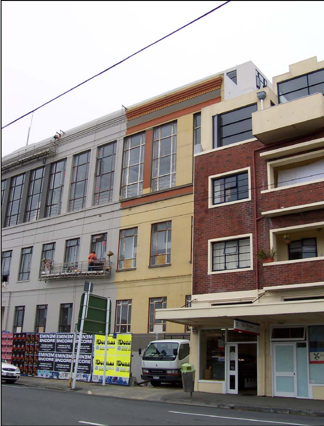
Restoration and repainting of the Willis St facade. Photo by Ann McEwan on 02.12.2004
