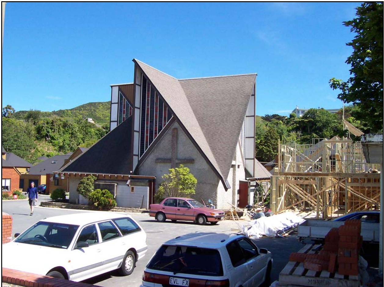
Futuna Chapel from Friend St with units under construction adjacent to the chapel. Photo by Ann McEwan on 30.11.2004.
