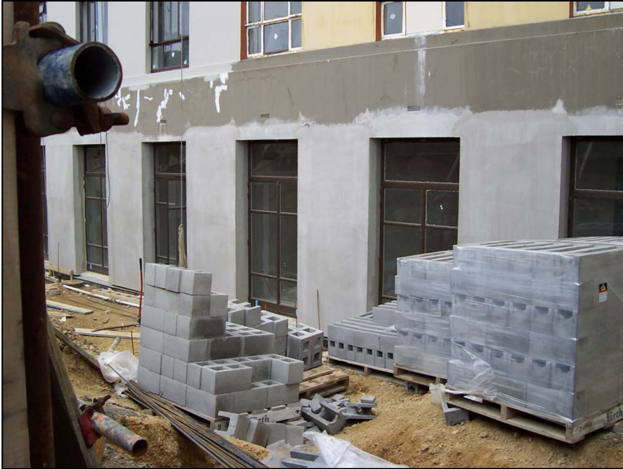
View of the work being undertaken at basement level. Photo by Ann McEwan on 02.12.2004.
