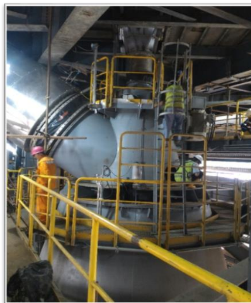
Figure 3. Photograph of Classifier – Coal Mill Measurement
