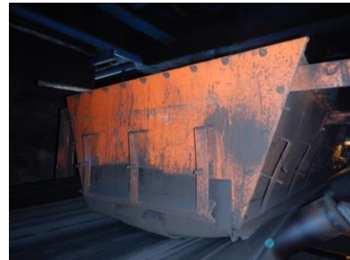
Figure 10. Tailbox extension at transfer point area
