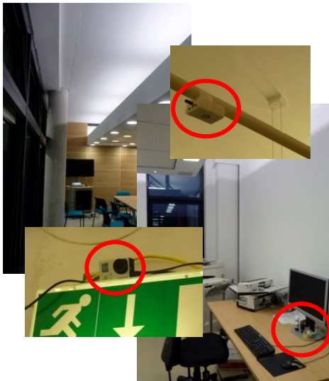
Figure 2: deployment of pervasive sensing within the Kingsgate building.
