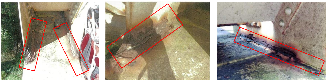
Fig. 2.1 Frequently corroded locations on steel truss bridges.
