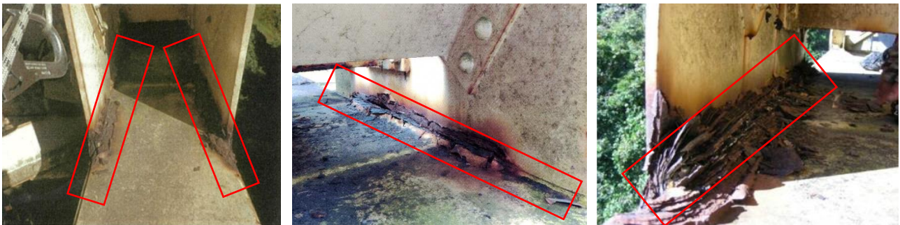
Fig. 1.2 Frequently corroded locations on steel truss bridges.
