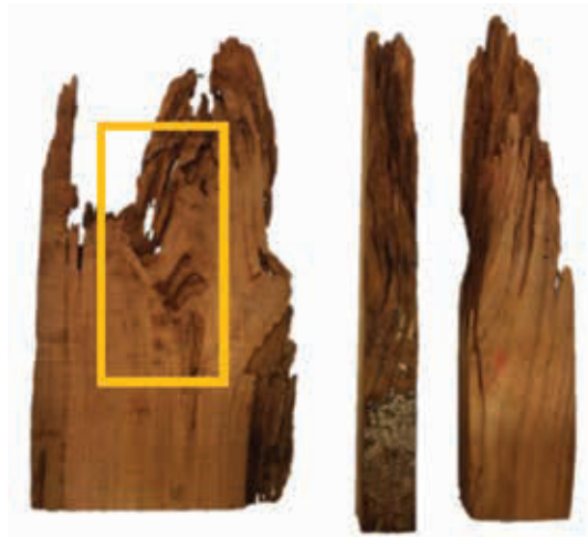
Figure 3. Longitudinal sections of beam heads showing the damage produced by large cerambycidae larvae, alternated with undamaged pieces. Larvae tunnels reaching the alburnum are visible amidst portions of undamaged wood.
