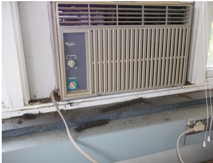
Figure 12: Window air conditioning unit (commonly found in older campus buildings) in one departmental repository
