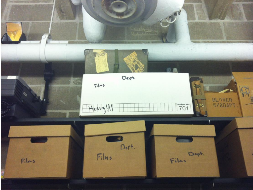
Figure 33. Examples of unique departmental films and video stored directly beneath building piping and conduit.
