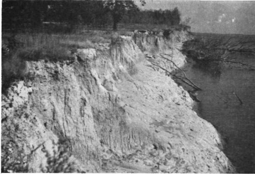
Figure 2. Wind-generated wave erosion in Carlyle Lake
