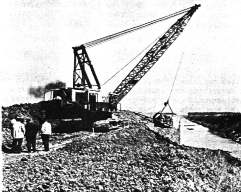
Figure 1. Modern dragline cleaning a drainage channel. (Courtesy of the Soil Conservation Service)
