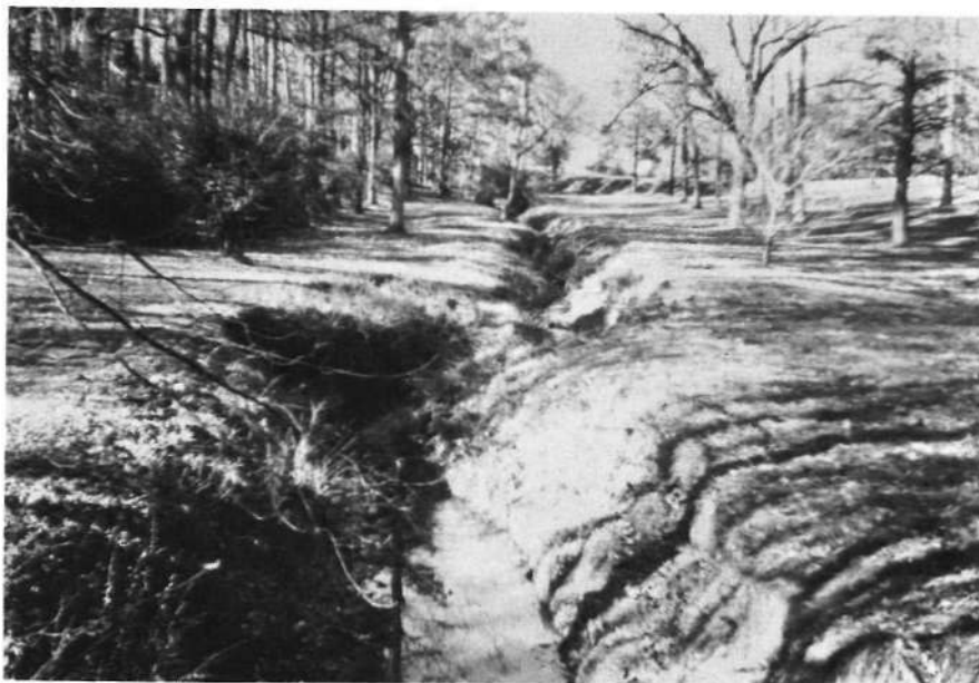
Figure 27. Open channel which is representative of most of the drainage in Third Fork basin
