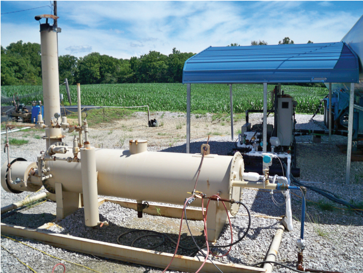
Figure 53 Natco 263,800 kJ/hr (250,000 Btu/hr) line heater. In-line heater's CO 2 inlet (right) frosted over; top of this line has Siemens pressure gauge/transmitter (small box with blue circle on casing) that is connected to the Globe Cast pressure control valve. In-line heater discharges to the injection line (blue line to right). Photo courtesy of Trimeric Corp.
