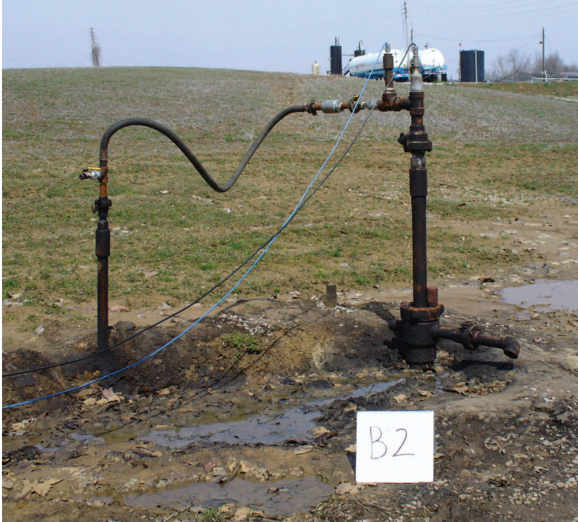
Figure 57 A typical production wellhead (right), IB-2 (B2), at the Bald Unit. The Bald Unit tank battery and CO 2 storage tanks are visible in the background. The cables emerging from glands on the wellhead are for pressure (black cable) and temperature (blue cable) gauges. Production flow line is to the left.
