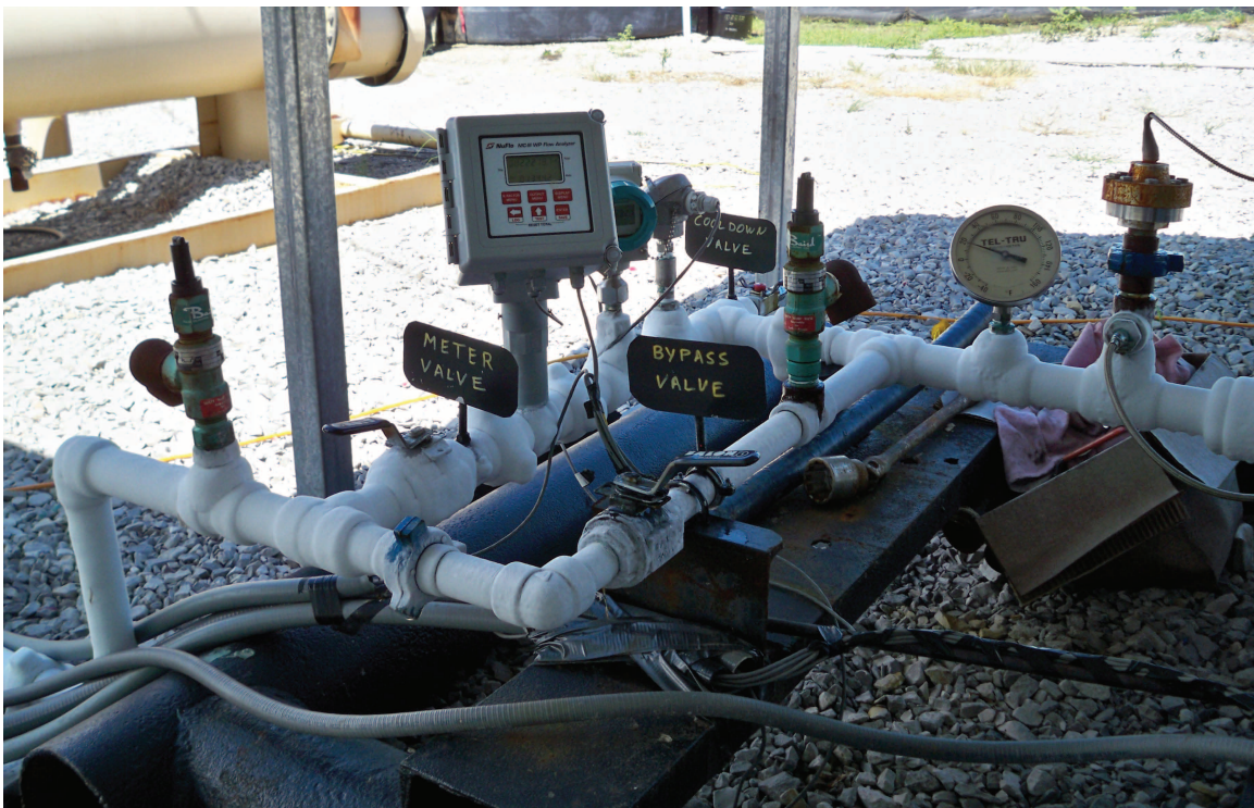
Figure 55 Cameron NuFlo liquid turbine meter (center, immediately behind “meter valve” sign) and Siemens pressure gauge (with blue cover, immediately behind NuFlo meter) in series on frosted line. In-line heater in upper left background. Tel-Tru mechanical temperature gauge at right is connected to pump discharge line. Photo courtesy of Trimeric Corp.
