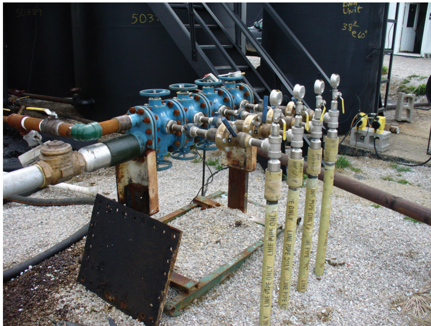
Figure 13 Production manifold at Bald Unit tank battery. Four vertical production flow pipes are in the foreground at center. Mani-Flo dual valve flow diverters are painted blue. Baker chokes (brass with blue handle) are between the flow diverters and the stainless-steel tees. The tees are topped with mechanical pressure gauges (backs shown). The large gray line to left leads to the gas-liquid separator.
