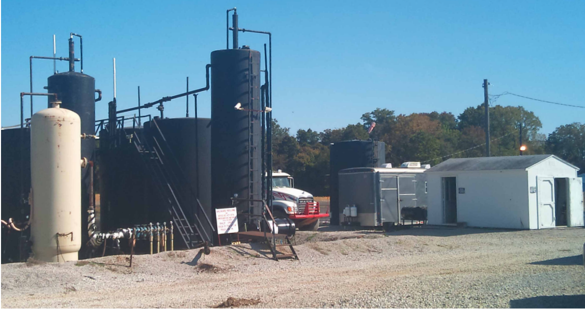
Figure 4 The tank battery at Mumford Hills Field, including tanks and pump house. Tanks are to the left, and the water injection equipment and accessories are in the white pump house at right.
