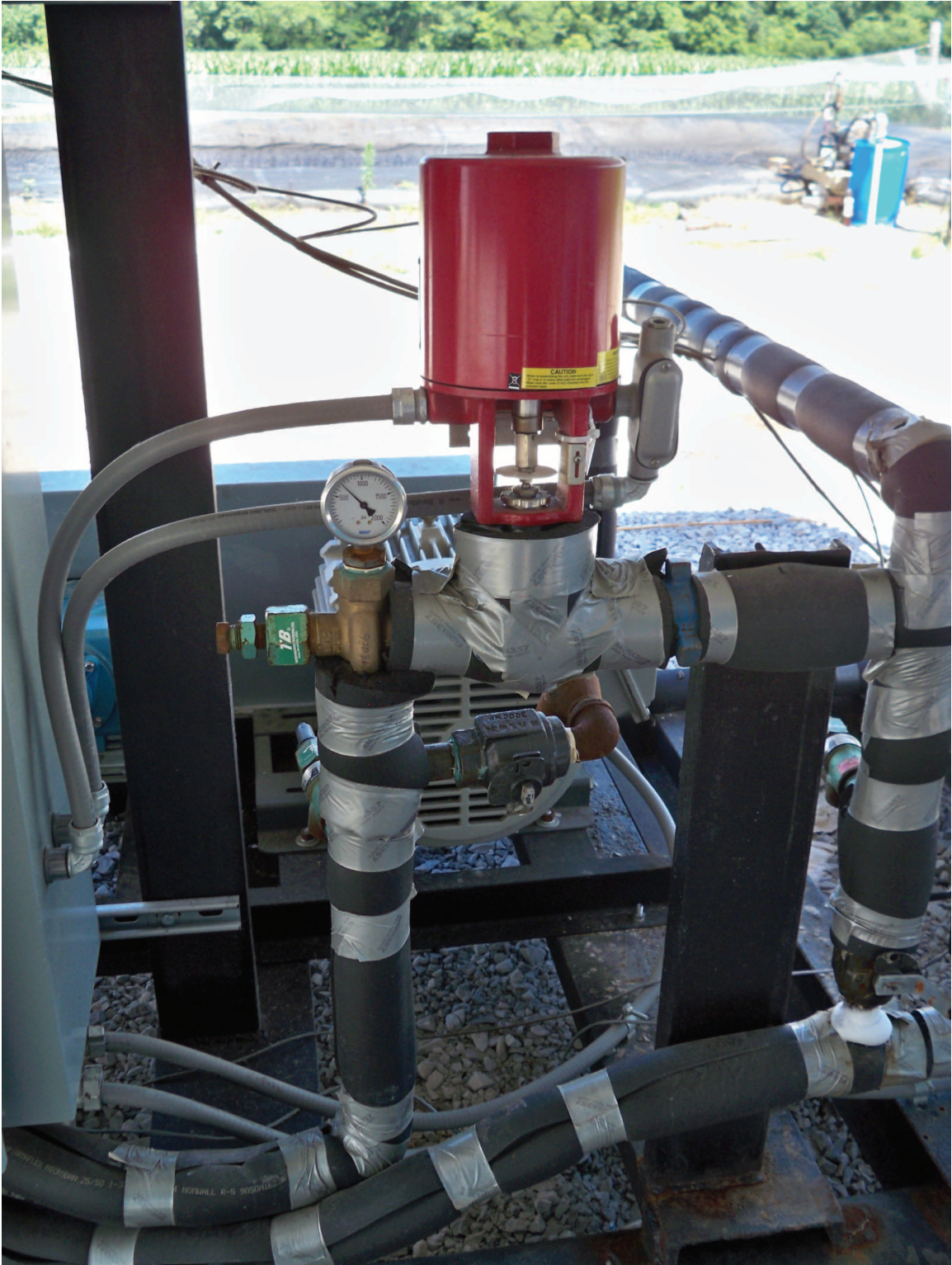
Figure 52 Globe Cast (BadgerMeter, Inc.) pressure control valve (red object at upper center) on return line between discharge of main pump and storage tank. The red casing conceals an electric actuator. The valve is below the actuator and is covered with black neoprene and gray duct tape. Photo courtesy of Trimeric Corp.
