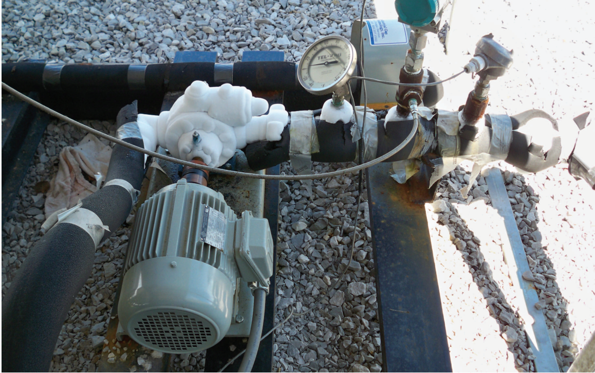
Figure 48 Booster pump (frosted over) and motor. The circular dial at the upper center of the photo (labeled Tel-Tru) is a manual temperature gauge. A Siemens pressure gauge (green-blue back, partially out of frame at upper right of photo) is located to the right of the manual gauge. Lines are covered with neoprene pipe insulation. The storage tanks are to the right; the main pump is to the left. Photo courtesy of Trimeric Corp.
