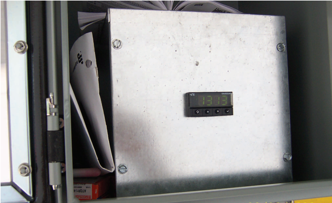
Figure 54 Omega pressure controller panel cover and housing at Sugar Creek site with pressure reading shown. Photo courtesy of Trimeric Corp.
