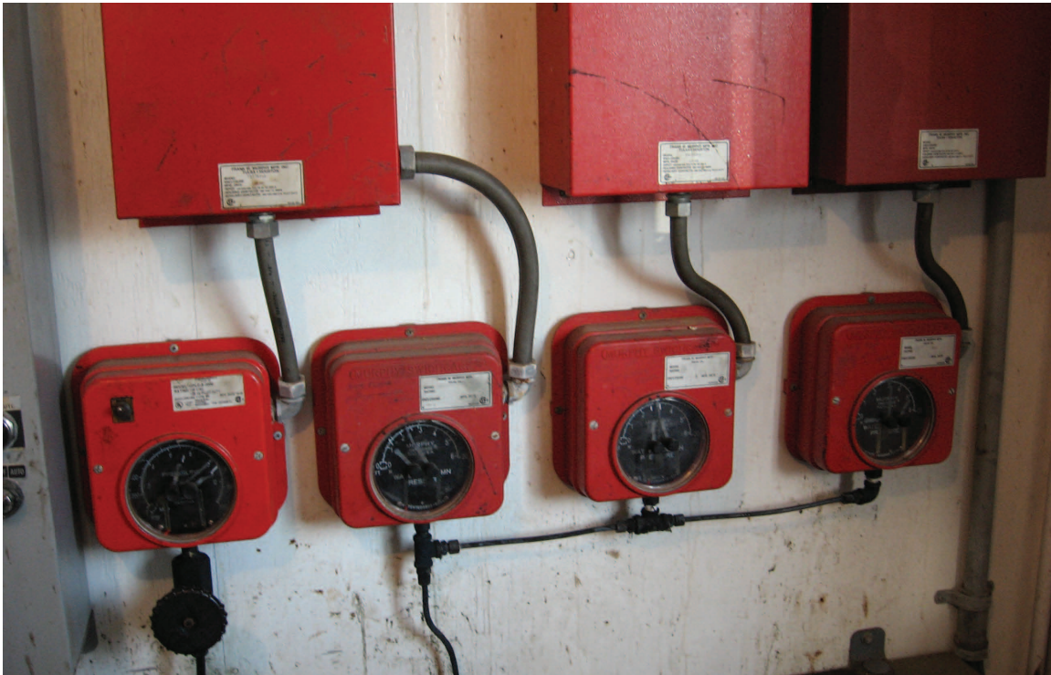
Figure 15 Example of control panels for water injection equipment in the Bald Unit pump house. (The photograph is from Sugar Creek Field.)
