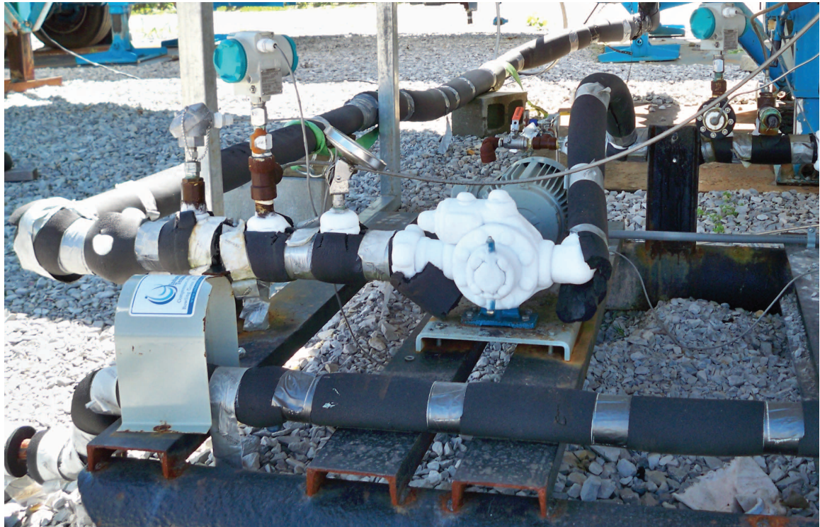
Figure 49 Injection pump skid at the Bald Unit tank battery. Frosted-over booster pump and motor seen in Figure 48 are visible at center. CO 2 tank supports are visible in background. Photo courtesy of Trimeric Corp.
