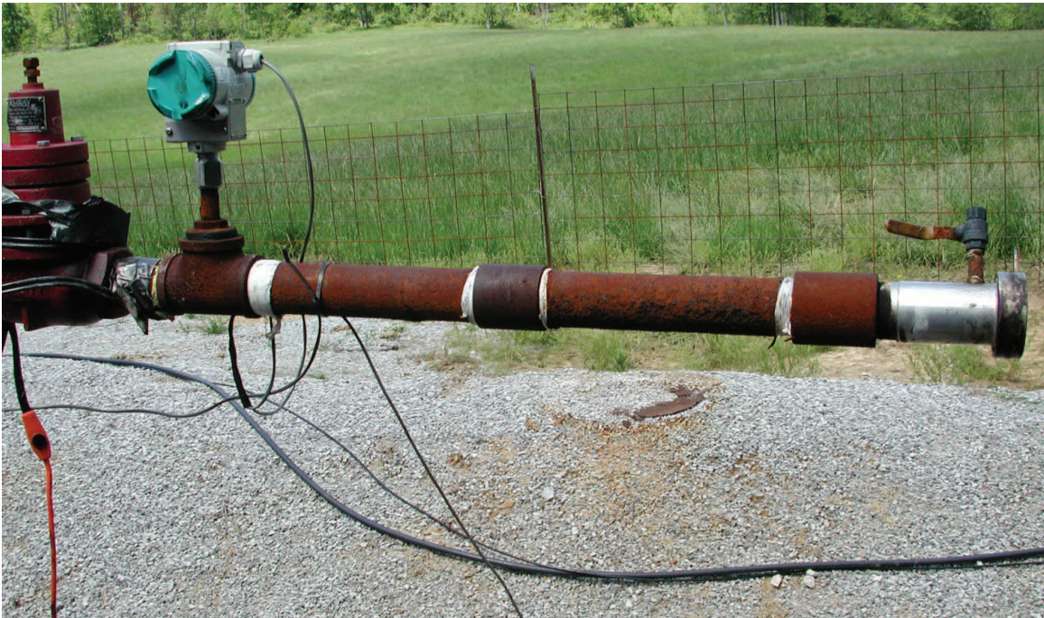
Figure 17 Teledyne Merla orifice well tester (aluminum pipe to right) attached to the liquid-gas separator at the Sugar Creek Field tank battery (a photograph of the well tester at the Bald Unit tank battery was not available). A Siemens electronic pressure transducer (blue cover) is shown on the left side of the figure.
