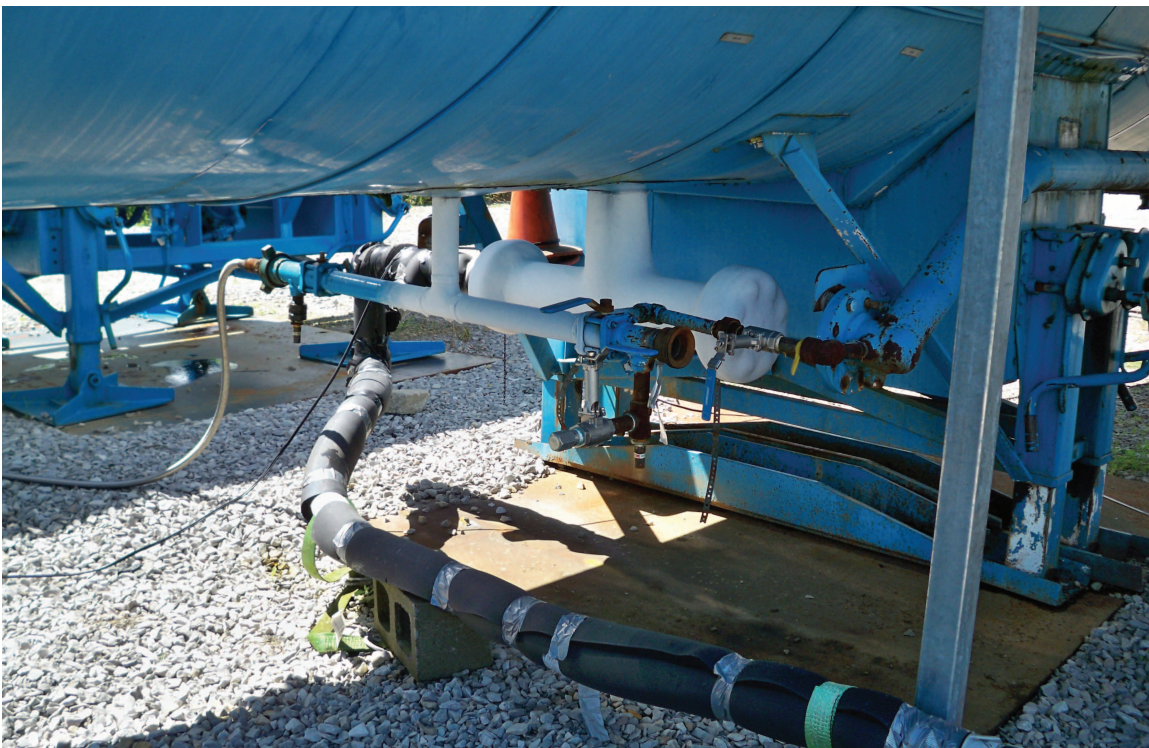
Figure 47 Connection line between CO 2 storage tank and injection equipment. Photo courtesy of Trimeric Corp.
