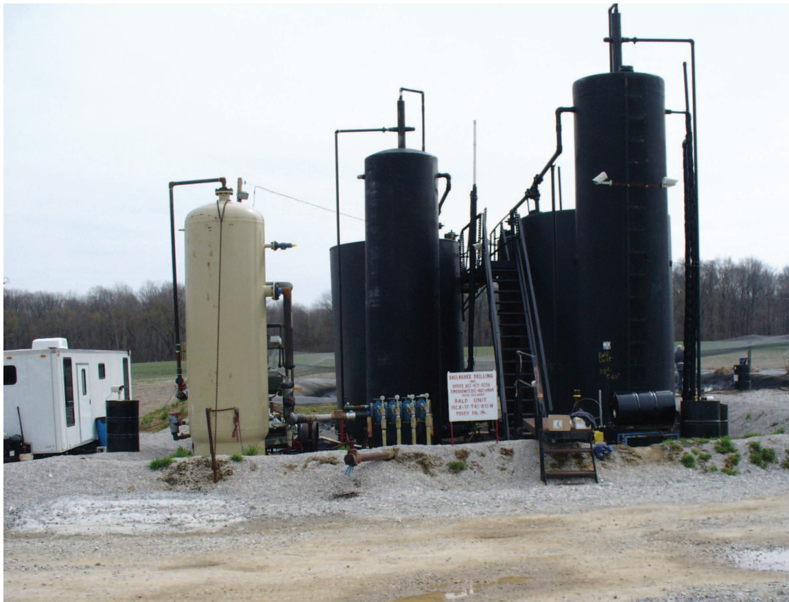
Figure 14 Bald Unit tank battery. The light-colored tank at left is the gas-liquid separator. The taller black tank behind the production manifold is the Natco “gun barrel” oil-water separator. The shorter black tanks behind the gun barrel are oil tanks. The second gun barrel at right was not used in the pilot project; BU-4 production was isolated from the pilot production and was sent to this gun barrel and to separate oil tanks.
