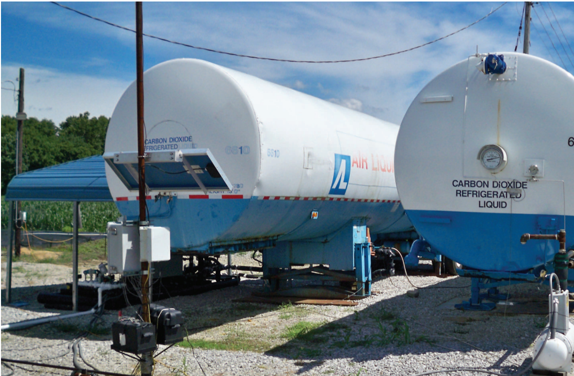
Figure 46 Portable Air Liquide CO 2 storage tanks. Tank capacity is 55 tonnes (60 tons) of CO 2 . Photo courtesy of Trimeric Corp.
