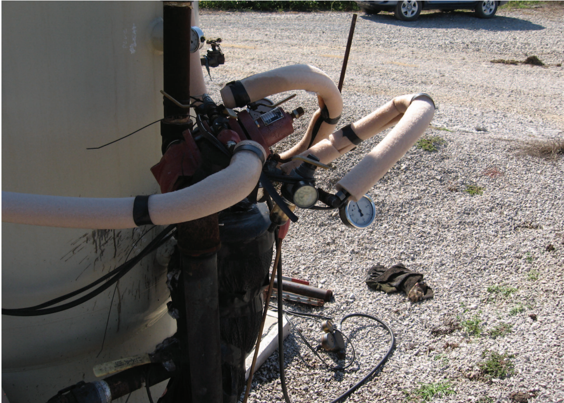
Figure 16 Kimray cast iron back-pressure gas regulator attached to gas separator at the Bald Unit tank battery. Well tester (see Figure 17) is visible immediately above and to the left of the gas regulator.
