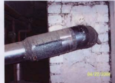
Figure 6 - Gap in furnace flue in basement.
