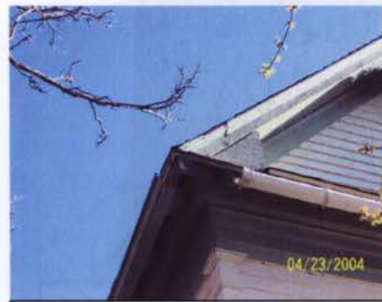
Figure 3 - Home with incomplete gutter system
