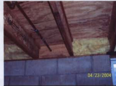
Figure 2 - Uninsulated band joist
