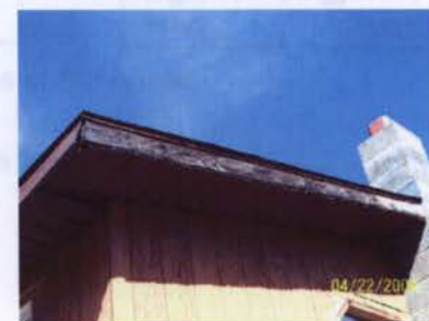
Figure 3 - Missing fascia on gable end.
