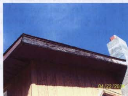
Figure 8 - Missing fascia at gable end
