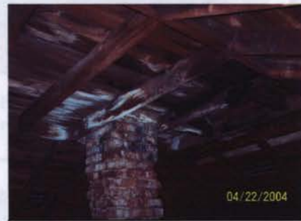
Figure 1 - Water damage under roof and on chimney due to roof
