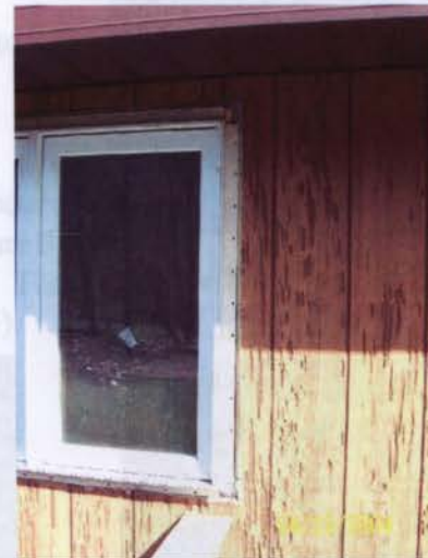
Figure 2 - Missing trim around windows.
