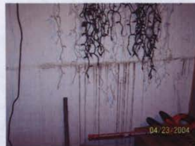
Figure 2 - Leaky cold joint in basement wall.
