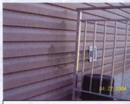
Figure 6 - Algae growing on north face
