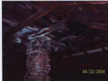
Figure 5 - Water damage under roof.
