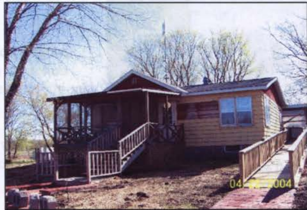
Figure 4 - Home with gutter over doorway; home was raised to improve the site drainage.
