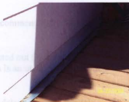
Figure 9 - Poorly installed flashing collects water.
