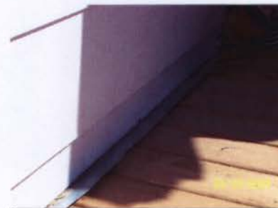
Figure 3 - Poorly installed flashing.
