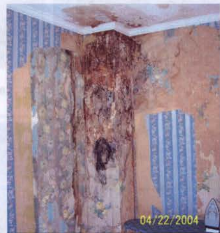
Figure 2 - Water damage from leaky roof around chimney
