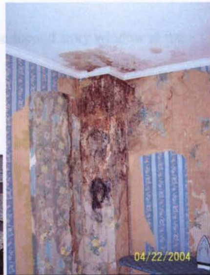
Figure 2 - Moisture damage on walls due to roof leak.
