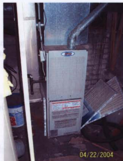
Figure 11 - Uncapped filter slot at furnace
