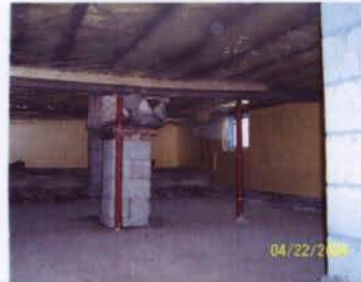
Figure 2 - Sagging beam in crawl space.
