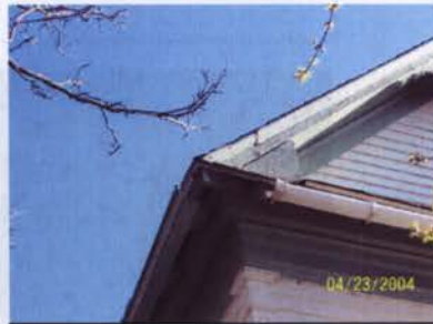
Figure 2 - Missing section of gutter and downspout.
