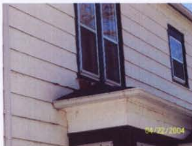
Figure 4 - Water damage below 2nd story windows.
