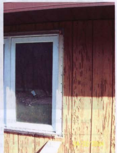
Figure 7 - Missing trim around windows
