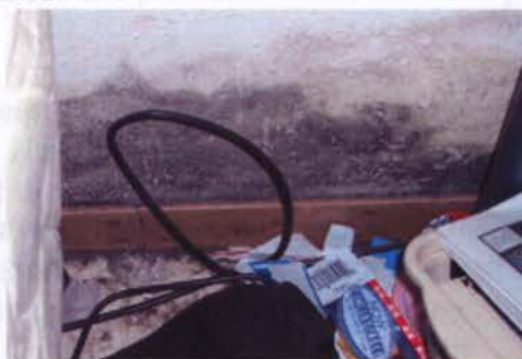
Figure 4: Mold at the bedroom base of exterior wall
