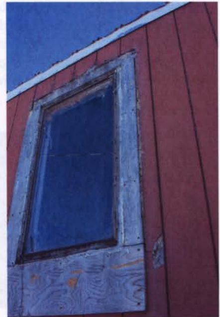
Figure 8: No overhang and poor window flashing caused water damage around several windows.
