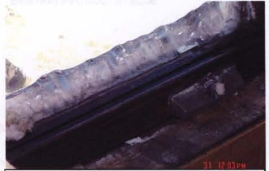
Figure 11: Ice on interior window indicate thermal bridging at the frames.
