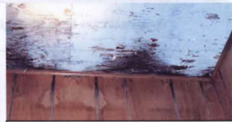
Figure 2: Mold at entry door ceiling
