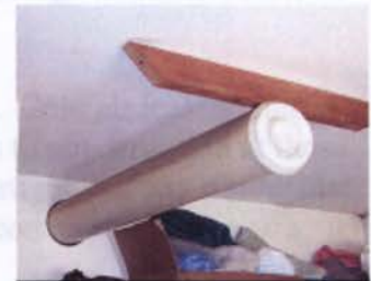
Figure 11: Fresh air vent outlet
