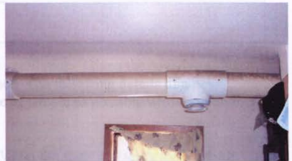
Figure 12: Existing ventilation ductwork.
