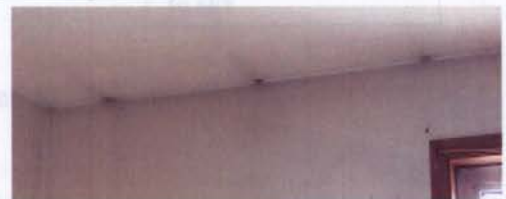
Figure 5: Mold at wall to ceiling juncture at truss bearing locations
