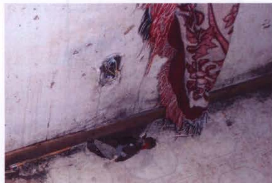
Figure 14: Water damage at base of exterior wall and the electrical outlet.
