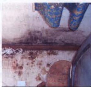
Figure 6: Mold at wall base
