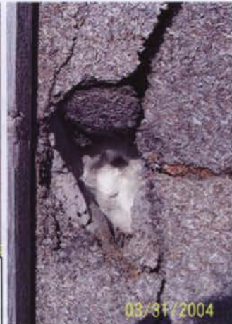
Figure 5: Hole through siding
