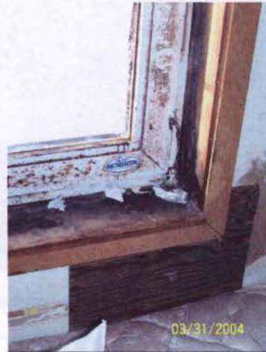
Figure 4: Condensation and mold on window frames
