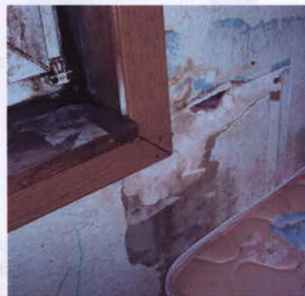
Figure 5: Window sill mold and wall deterioration
