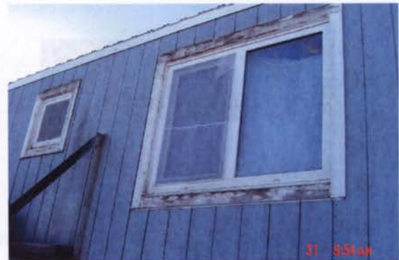
Figure 1: No roof overhang, and poorly sealed and flashed windows, has led to water intrusion.
