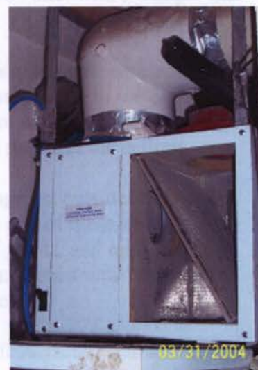
Figure 12: Interior of fresh air filter
