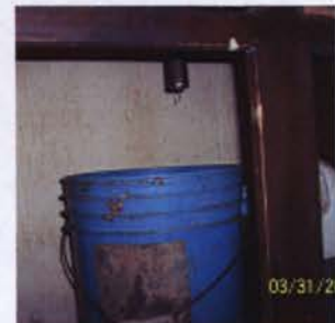
Figure 9: Bucket beneath vanity
