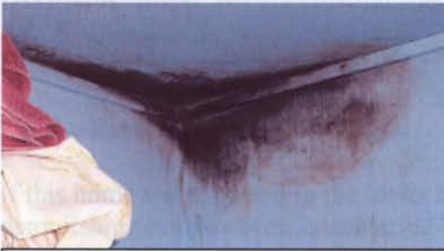
Figure 2: Mold at exterior corner
