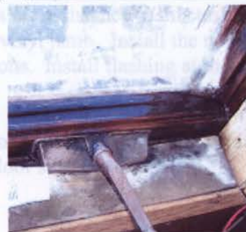
Figure 5: Ice and water on window sill
