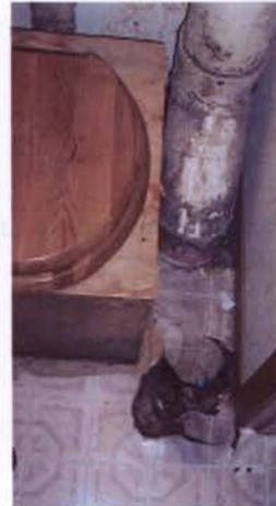
Figure 8: Hole through floor
