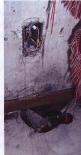
Figure 12: Nonfunctioning outlet and a hole in the floor due to moisture
