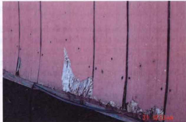
Figure 6: Deteriorated siding at the base of exterior wall.
