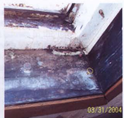
Figure 8: Moldy window sill
