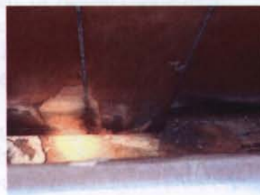
Figure 2: Moldy base of paneling behind a bed
