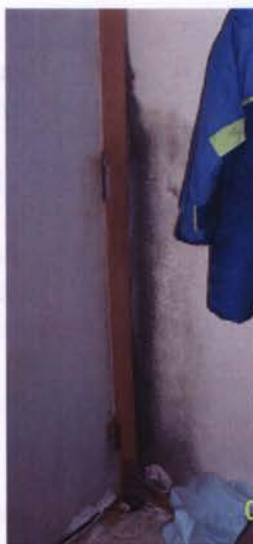
Figure 2: Mold at entry door
