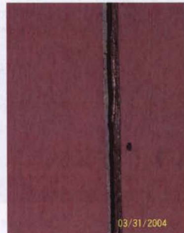
Figure 7: Gaps in siding,
