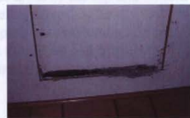
Figure 4: Mold at attic access hatch
