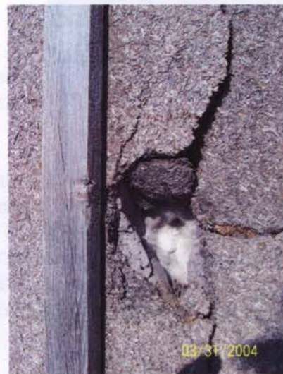
Figure 5: Hole in exterior cladding.
