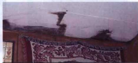
Figure 3: Mold at bedroom wall to ceiling junction
