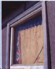
Figure 3: Gaps between window trim and siding
