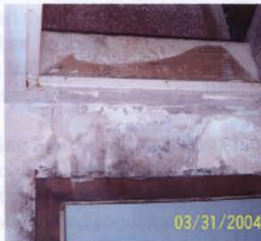
Figure 2: Mold at the front entry door
