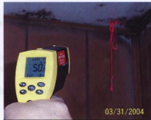
Figure 6: Cold exterior corner
