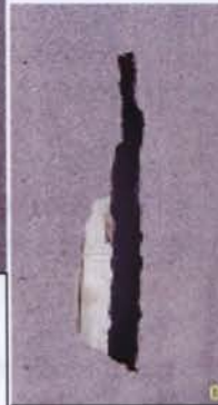
Figure 4: Hole in exterior sheathing
