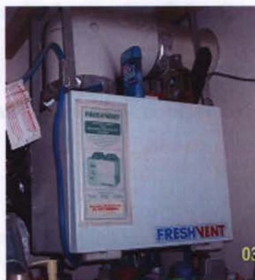
Figure 11: Fresh air system
