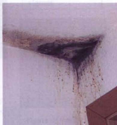
Figure 3: Mold at the bedroom wall to ceiling corner
