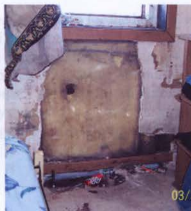
Figure 7: Missing drywall & hole in floor next to wall
