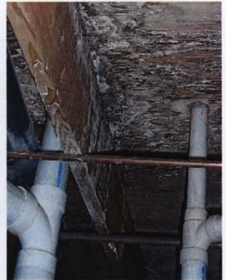
Figure 8. Plumbing - Leaks from the fixtures above these plumbing drains have led to severe deterioration of the floor deck and floor joists.
