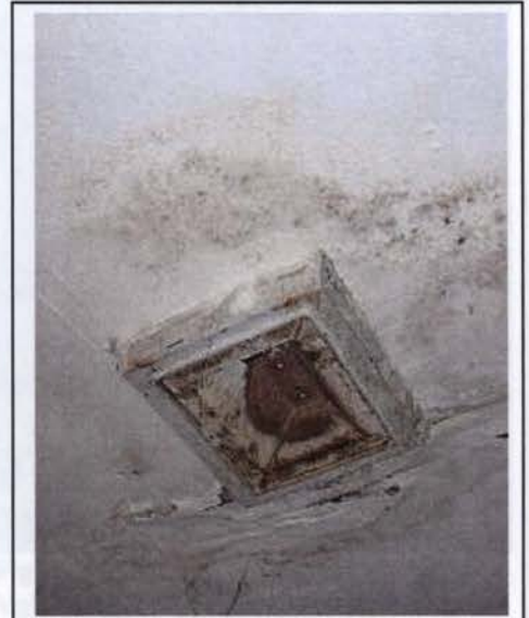
Figure 10. Exhaust Ventilation - Poor installation of the exhaust fan led to water damage in the area of the fan.
