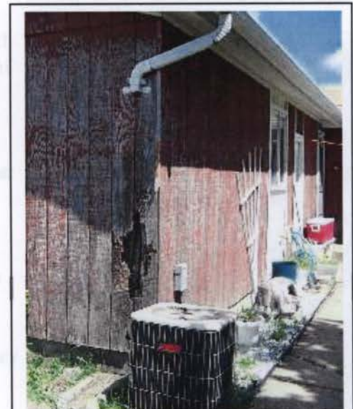
Figure 5. Gutter System - The missing downspout has led to severe rotting of the siding materials.
