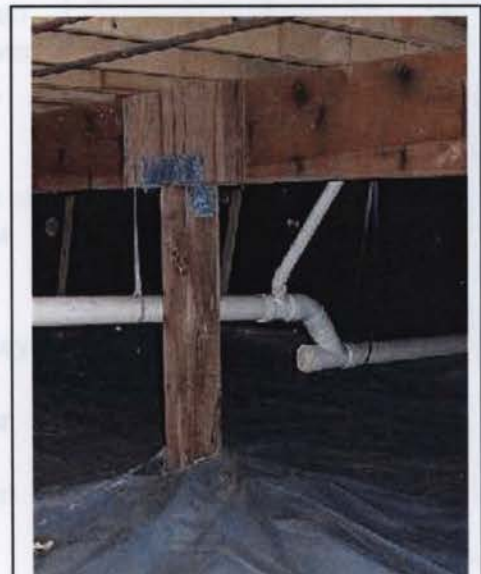
Figure 7. Basement and Crawl Space - The ground cover in the photo is necessary to prevent evaporation of water from the soil beneath.
