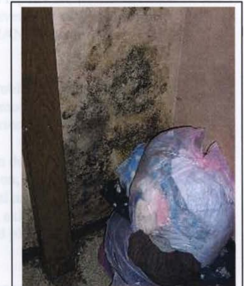
Figure 11. Exterior Wall/Ceiling - The combination of cold surface temperatures and high humidity lead to the class of problems called condensation problems.
