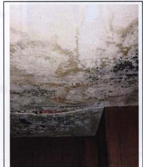
Figure 6. Leaks from Exterior - A roof leak has caused this severe deterioration of the ceiling materials.
