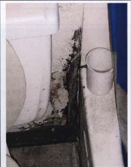
Figure 9. Bathroom - The wallboard between the tub and the toilet is a common site of deterioration.
