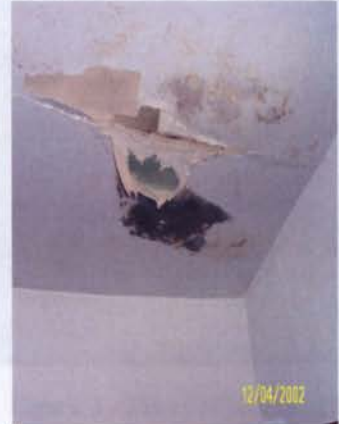
Figure 4 - Lower Level Bathroom Ceiling
