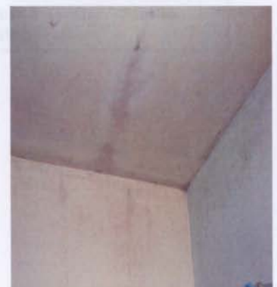
Figure 3 - Area above upstairs bathtub
