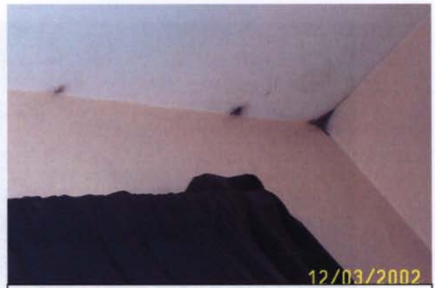
Figure 4: Mold growth at exterior wall/ceiling juncture
