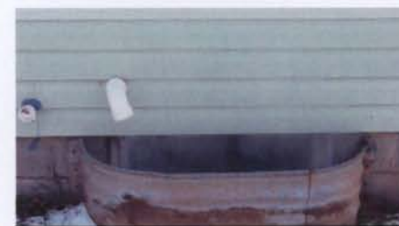
Figure 4 - Furnace Exhaust into Window Well
