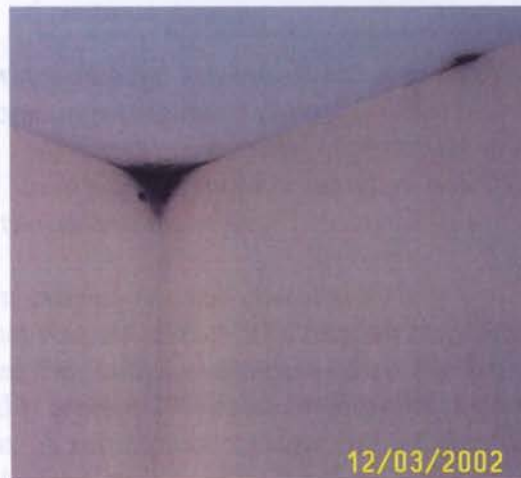
Figure 3: Mold growth at exterior wall/ceiling juncture
