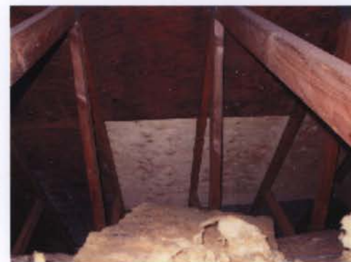
Figure 3 – Dark attic sheathing affected by crawl space water. Note new sheathing panel.
