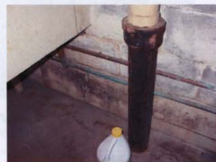
Figure 2 - Discoloration at Base of Basement Wall
