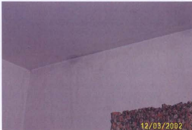
Figure 5: Water staining at wall/ceiling junction.
