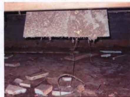
Figure 2 – Return Air Open to Crawl Space
