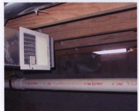
Figure 3 - Heating Register Proximate to Crawl Space Vent
