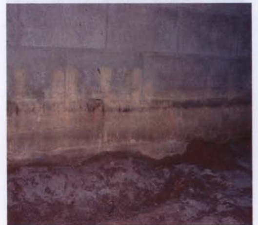
Figure 2 - Water Line on Block Walls
