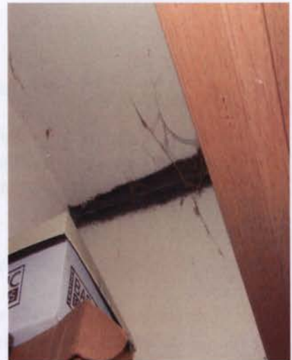
Figure 1 - Closet Exterior Wall to Ceiling Junction
