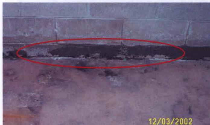
Figure 4: Crack between basement slab and foundation wall.
