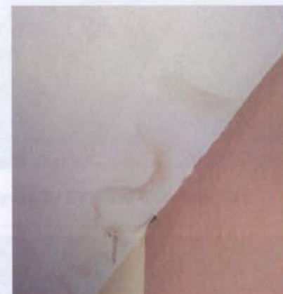
Figure 5 - Water Stains on Ceiling/Wall
