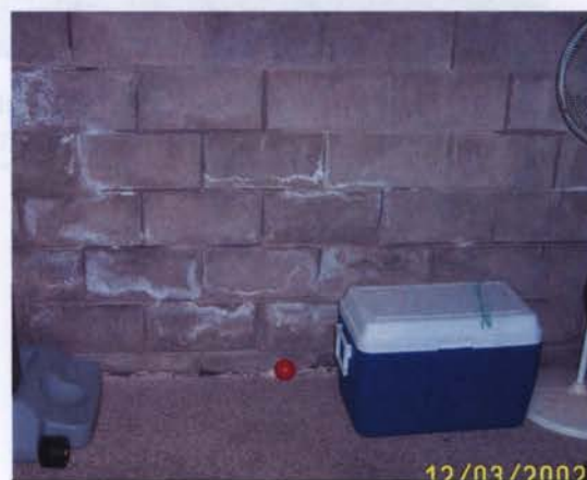
Figure 3: Staining from basement water entry.
