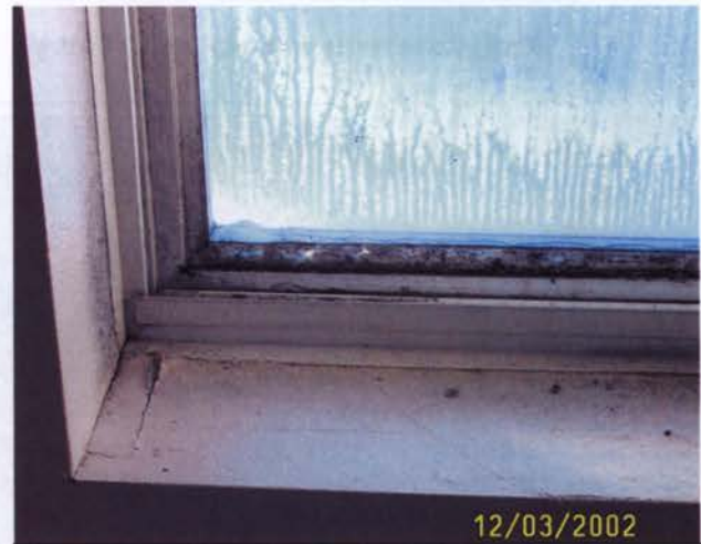
Figure 5: Window condensation, mold, and moisture damage
