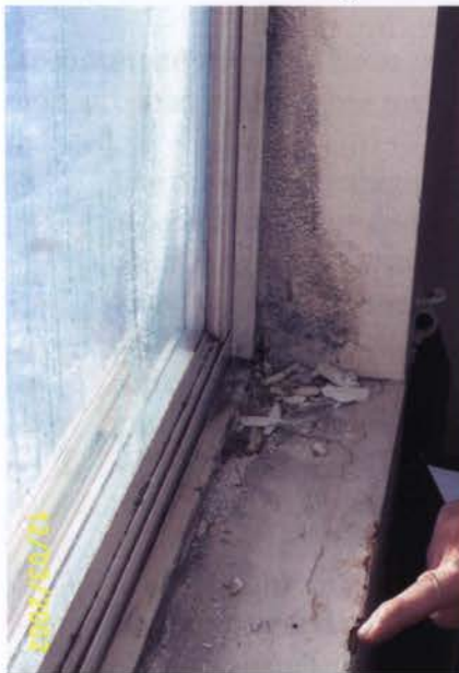
Figure 6: Window condensation, mold, and moisture damage
