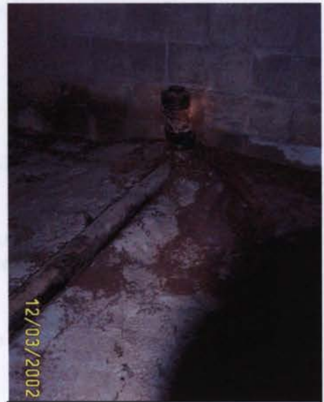
Figure 4: Sewer pipe in crawl space, possible leak.
