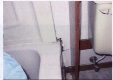
Figure 5 - Mold at Edge of Bathtub
