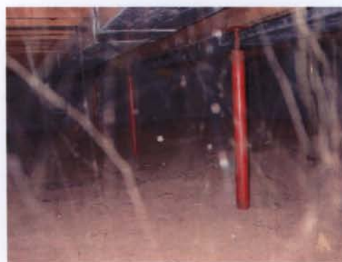
Figure 2 – Dry tall crawl space. However, cobwebs make the crawl space unpleasant to visit for maintenance and repair.
