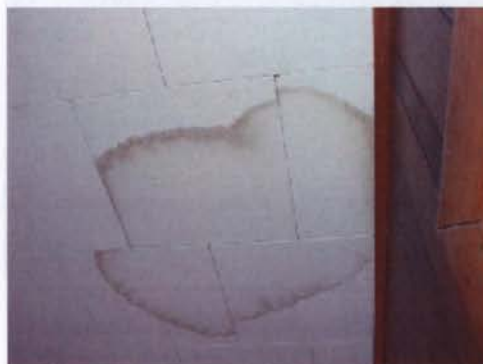
Figure 4 – Ceiling water spotting, a consequence of attic condensation.
