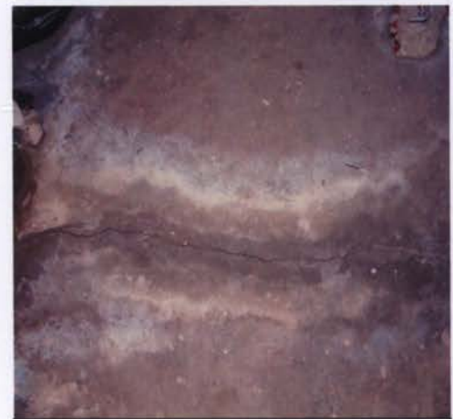
Figure 2 - Cracked Concrete Slab
