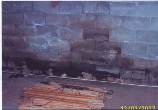
Figure 2: Wet foundation on the west foundation wall.
