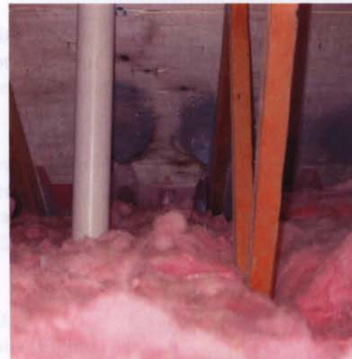
Figure 5 - Frost on Roof Sheathing
