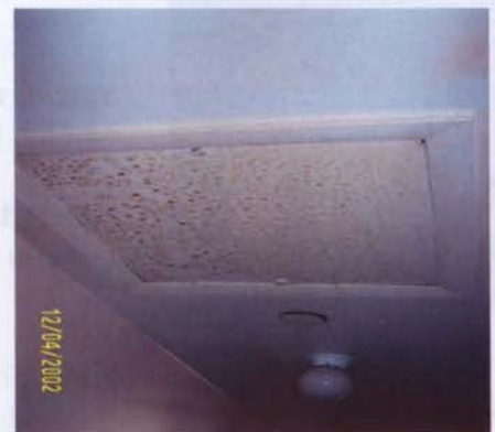
Figure 2 - Staining on Attic Access
