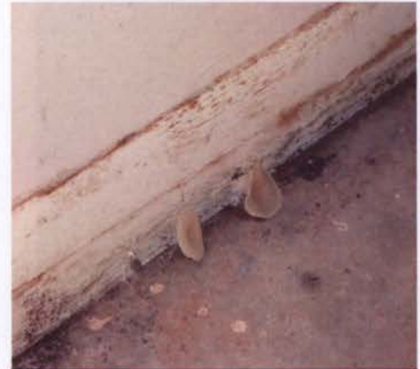
Figure 4 - Mushrooms at Baseboard
