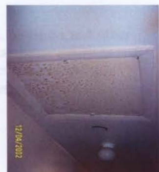
Figure 1 - Stained Attic Access Hatch
