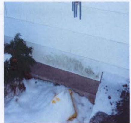
Figure 2 - Mildew on Siding
