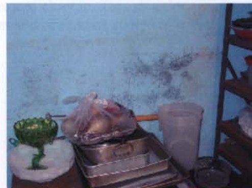
Figure 2 – Mold growth on shed walls as consequence of substandard cladding.
