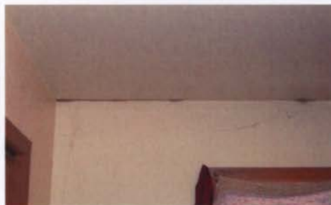
Figure 1 – Ceiling-wall joint showing darkening at truss locations.
