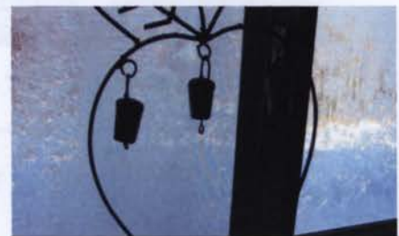
Figure 6 - Moisture on Plastic Window Covering
