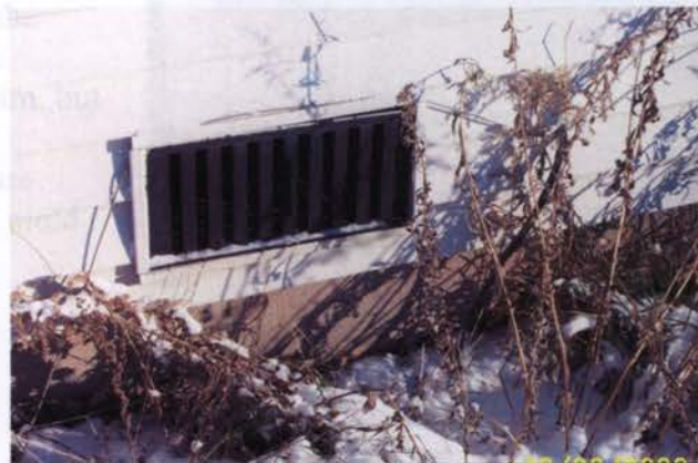
Figure 2: Crawl space vent
