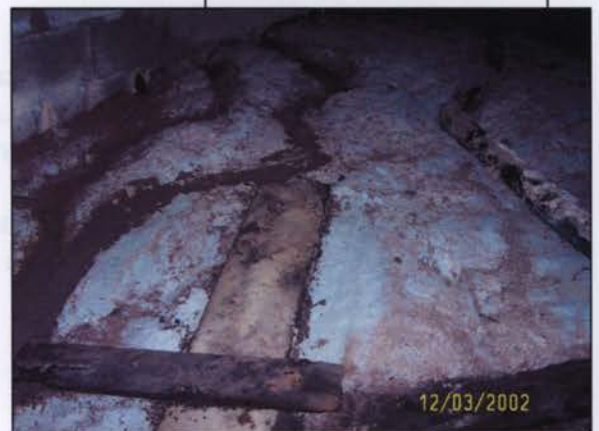
Figure 3: Crawl space. Note wood debris and signs of running water.
