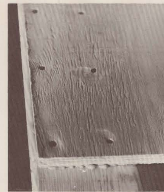
Nail Heads Buried in Plywood
