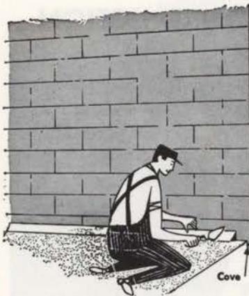
Leaks between foundation wall and footing can be eliminated by building a cove of quick-setting waterproofing cement.
