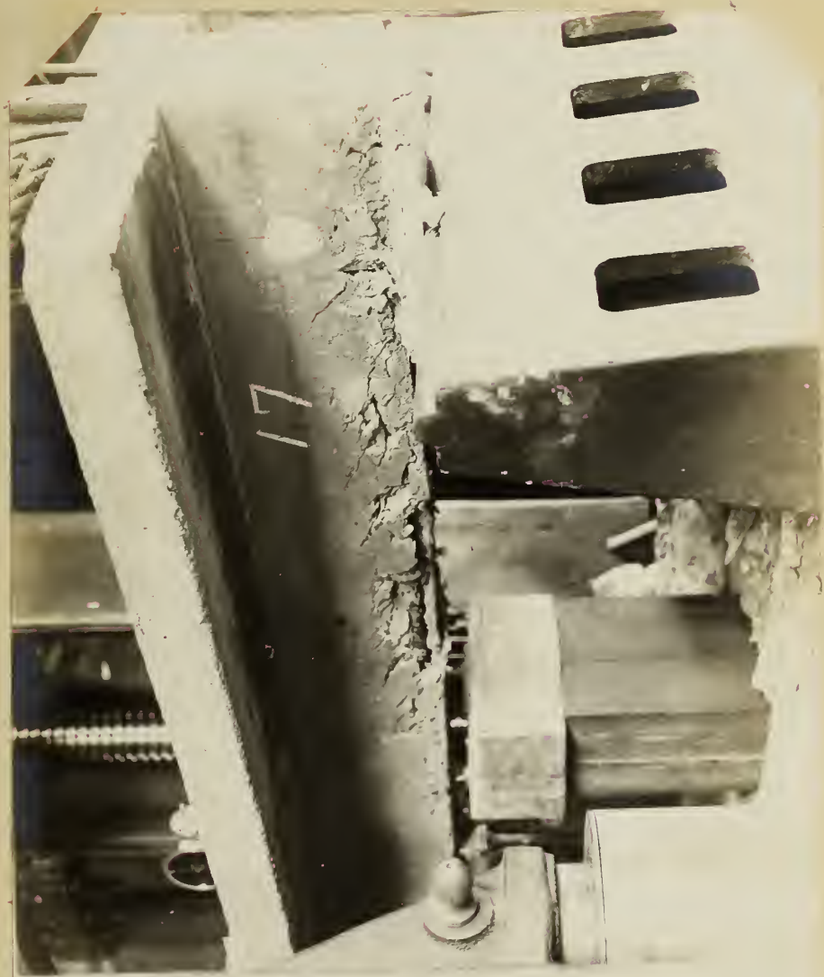
T-Beam No. 17 After Failure
