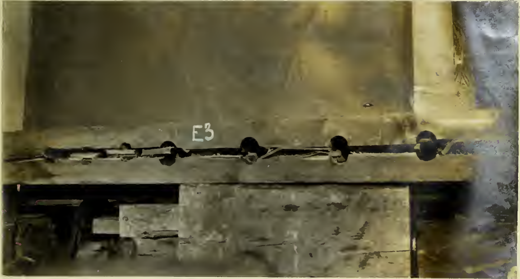
D 3, incorrectly marked E 3, showing condition of failure.
