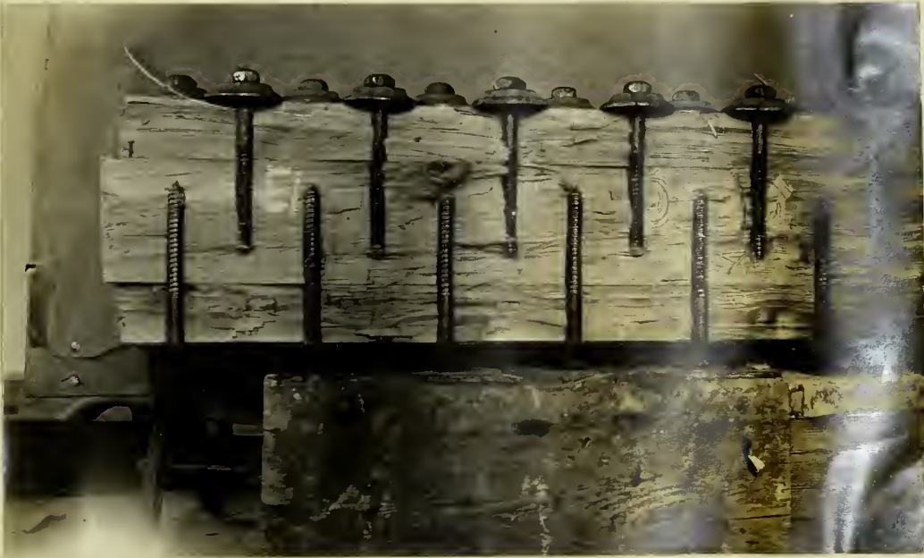
E 1 Showing condition of failure.
