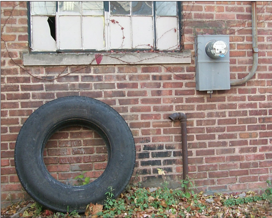
Figure 14 Vent pipe along building wall, indicating possible presence of an underground storage tank. Photograph by Daniel J. Adomaitis.
