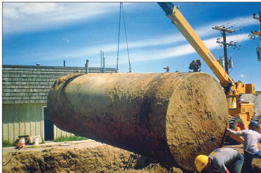
Figure 2 Unanticipated issues, such as undocumented underground storage tanks in state right-of-way, may cause construction delays and cost overruns. Photograph courtesy of U.S. EPA ( www.epa.gov/oust/graphics/trpics2.htm ).
