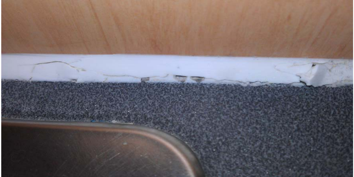
Figure 5-17 Image of the sealant breakdown on the equipment sink within the HSCTU.
