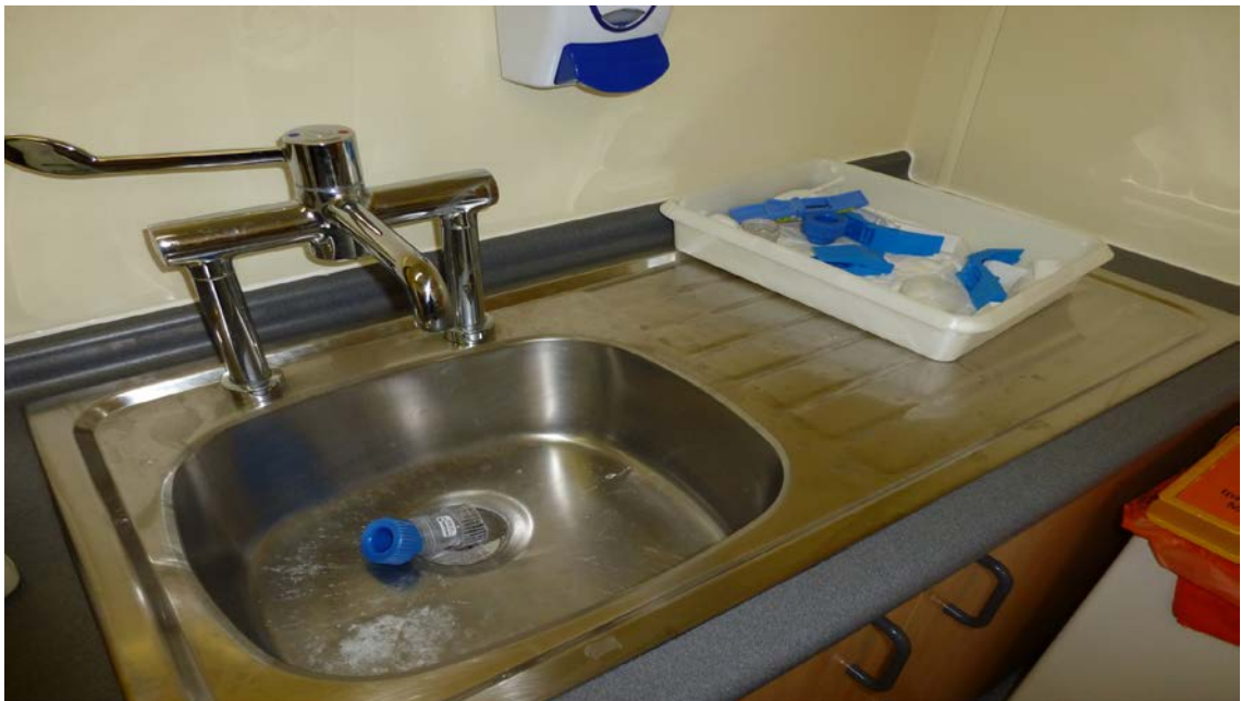
Figure 5-16 Photograph of the equipment sink within the HSCTU.
