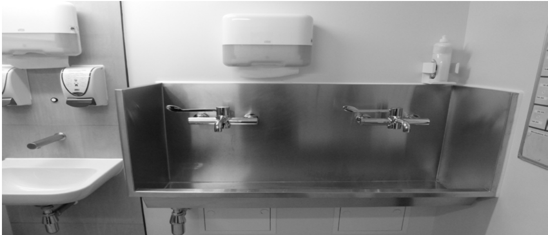
Figure 5-18 Replacement equipment sink fitted on the HSCTU at GOSH.
