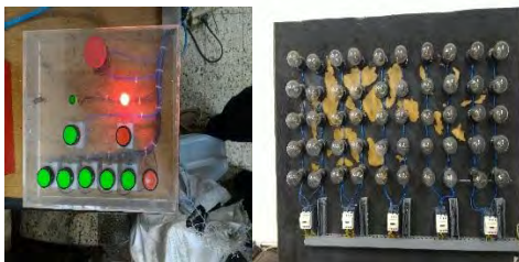
Figure 3. 5 Control Panel and Load
