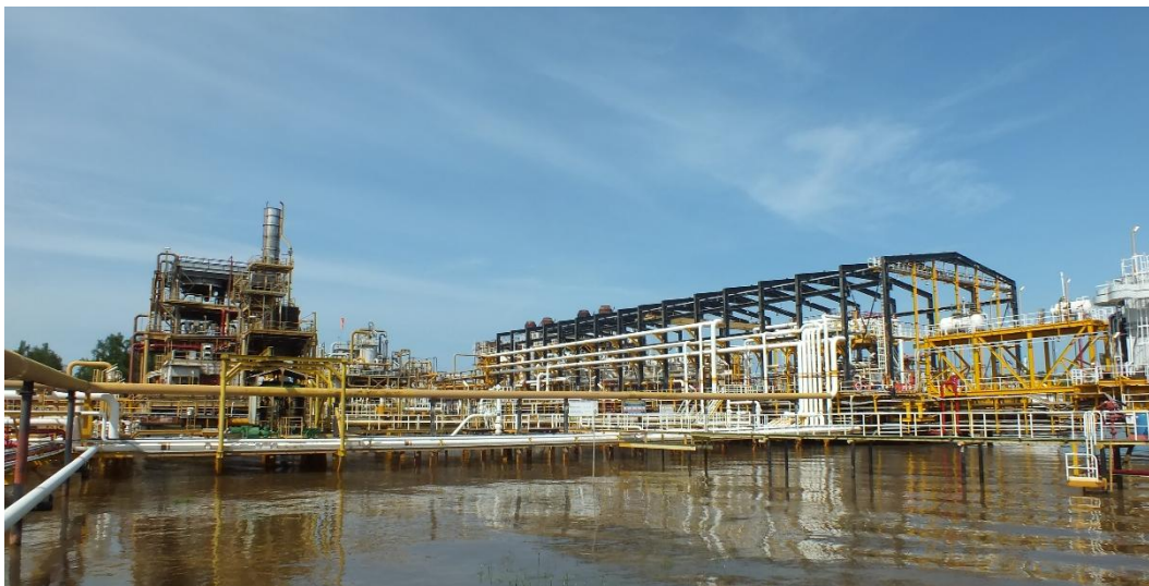
Figures 1.1 The installation of oil and gas processing area. This OGPA delivers production of hydrocarbon oil, gas and condensate.
