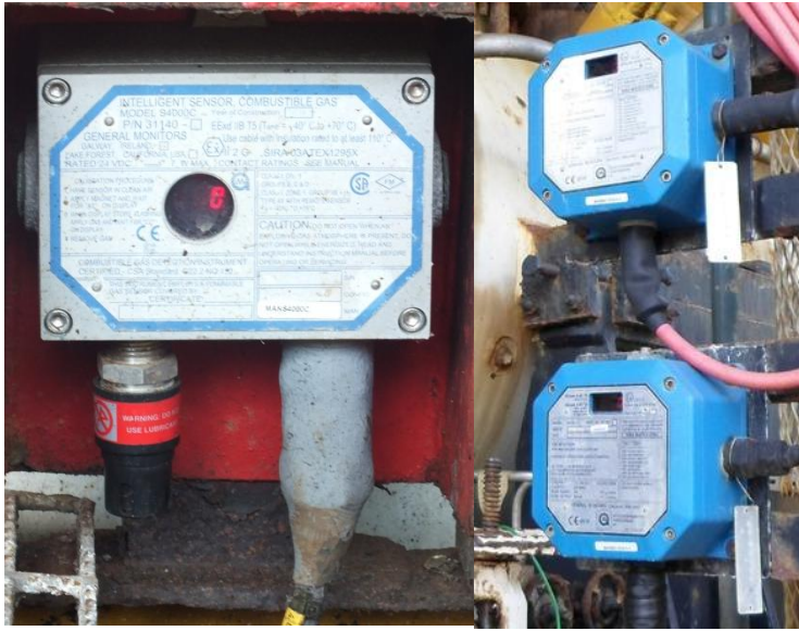
Figure 2.8. Installation of Catalytic gas detector. Based on its characteristic, this gas detector shall be placed in redundant configuration in one coverage area
