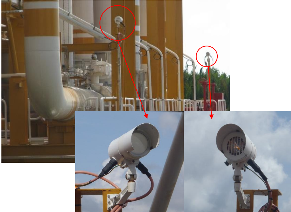
Figure 2.10. Installation of open-path infrared gas detector. It involves receiver and transmitter which detect gas concentration along the beam
