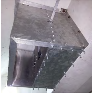
Figure 4.23. Modification of the Evaporator
