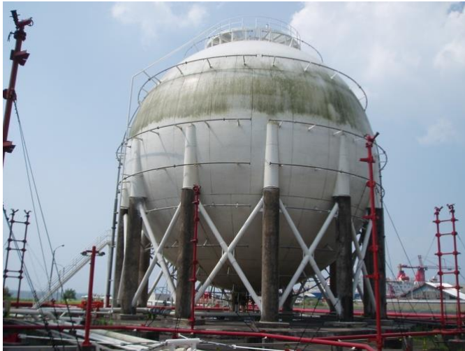
Figure 5.3 Spherical Storage Tank
