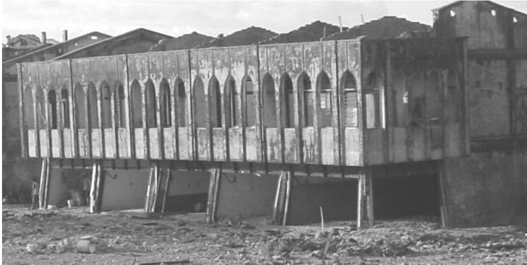
Figure 1-1 Soft story effect in a typical commercial building (Nias Earthquake, 2005)
