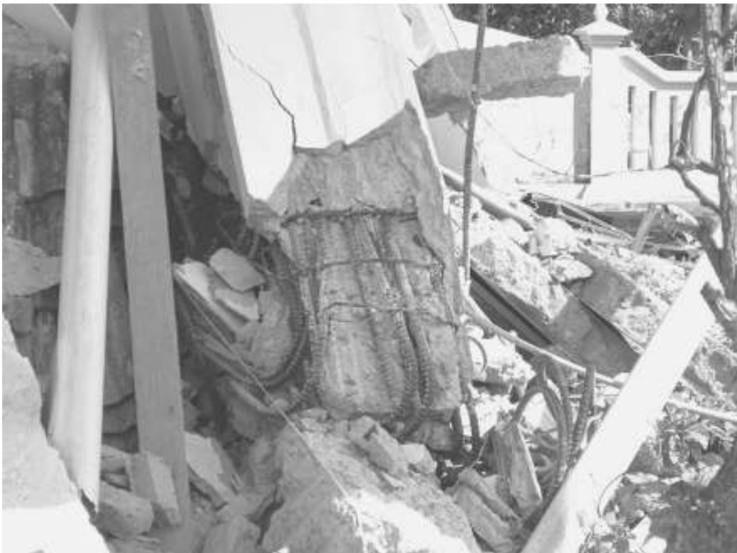
Figure 1-2 Inadequate transverse reinforcement in RC column (Yogyakarta Earthquake, 2006)
