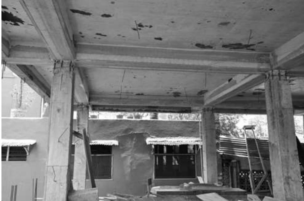
Figure 1-3 Inadequate columns' strength in joints (Padang Earthquake, 2009)
