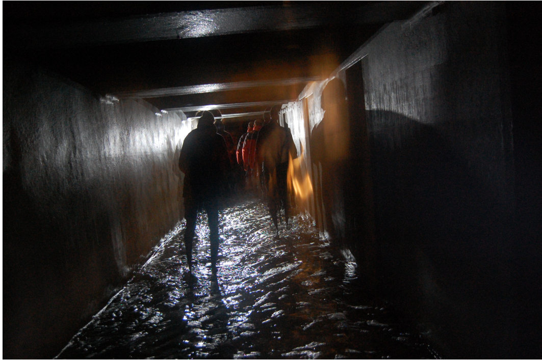
Figure 8.13. The flooded WWII air-raid shelter adjoining Dresdener Straße U-Bahn station. Source: Author 2008.
