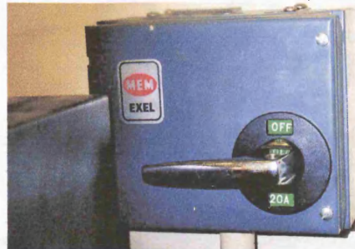
5) Above: Confining pump mains switch
