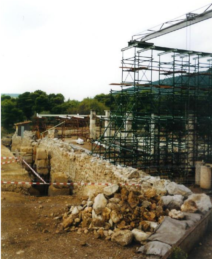
Figure 76b: works in the Avaton Stoa, for diagnosing the state of the structure and consolidating its surviving parts (source: Vacharopoulou -- personal photographs, 2002)
