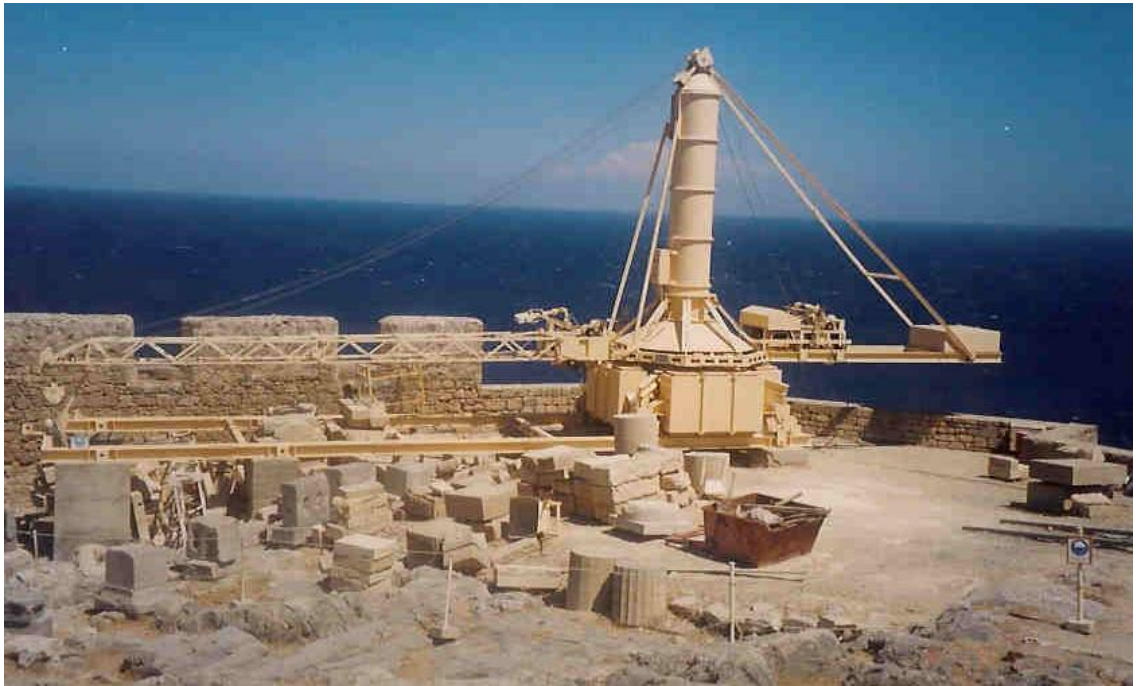
Figure 115a: the work-site near the stoa, inside the archaeological site (source: Vacharopoulou -- personal photographs, 2003).
