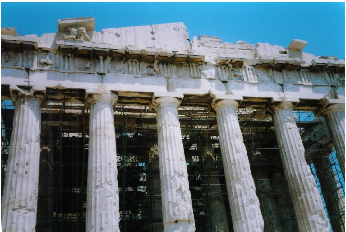
Figure 54b: close view of the west side of the Parthenon during anastylosis (source: Vacharopoulou -- personal photographs, 2002).
