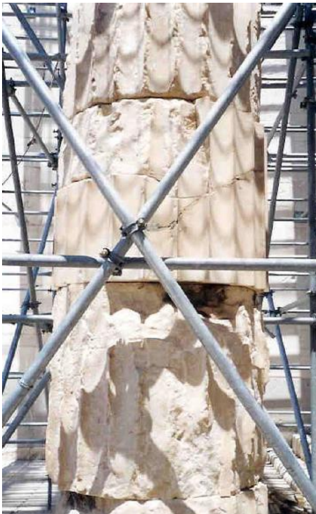
Figure 37a: example of shifted column drums (source: Vacharopoulou, personal photographs-- 2002).
