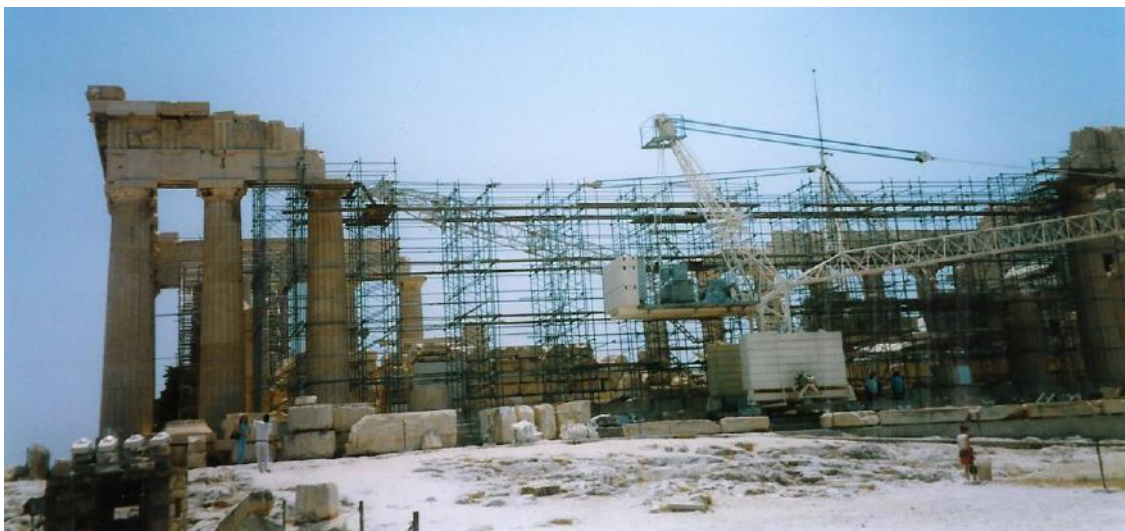
Figure 48: view of the north side of the Parthenon with the scaffoldings and the derrick crane (2003) (source: Vacharopoulou -- personal photographs, 2003).
