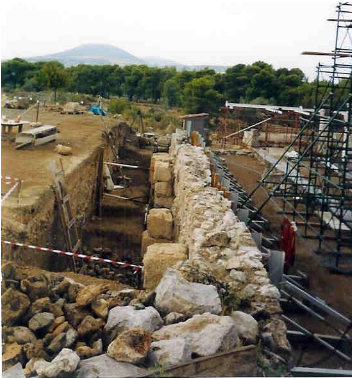
Figure 76a: works in the Avaton Stoa, for diagnosing the state of the structure and consolidating its surviving parts (source: Vacharopoulou -- personal photographs, 2002).
