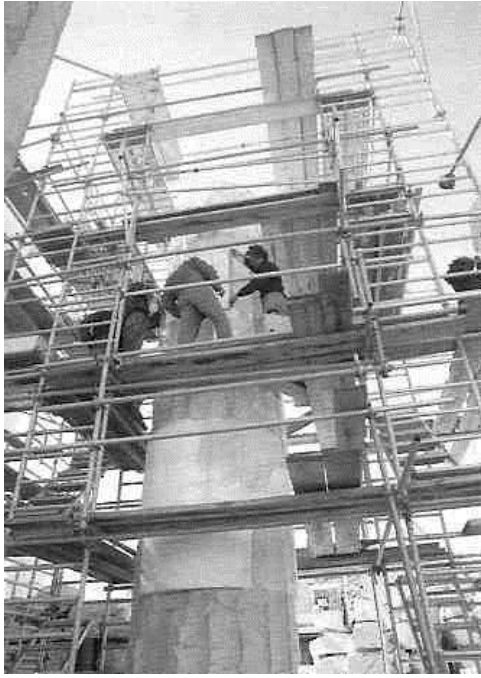
Figure 42: cutting the fluting on a column of the Parthenon pronaos (photo by Bouras, 2001) (source: SRAM 2002, 12).
