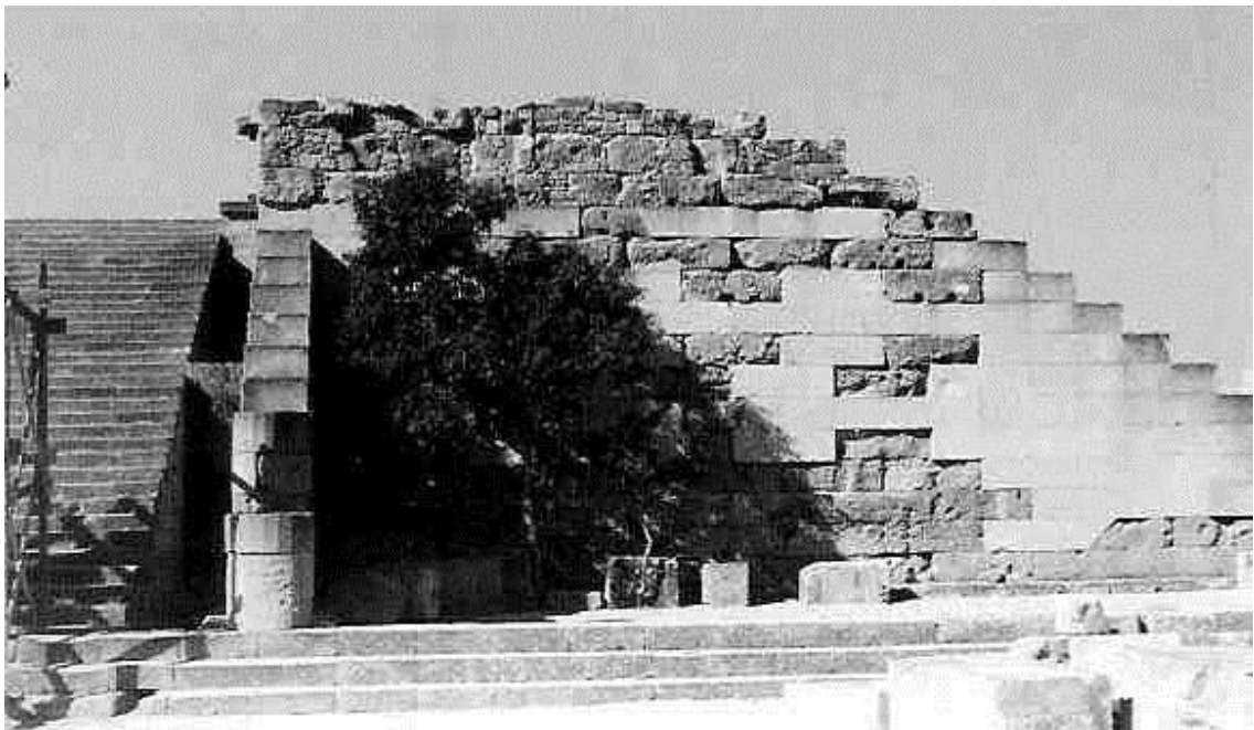
Figure 105: the back wall of the west side before the current interventions (1978) (source: Eleftheriou 2002h, 81).
