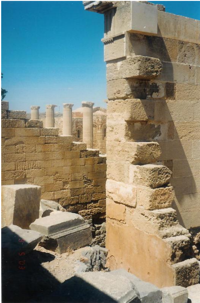
Figure 135a: view of the restored east wall of the stoa (source: Vacharopoulou -- personal photographs, 2003).
