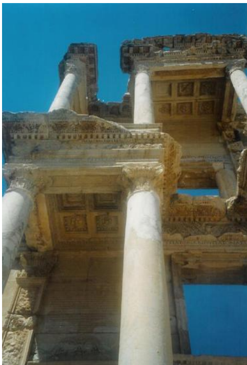
Figure 166c: close view of the restored façade of the Library, showing the colour of the new stone being suitable to the original (source: Vacharopoulou -- personal photographs, 2003).
