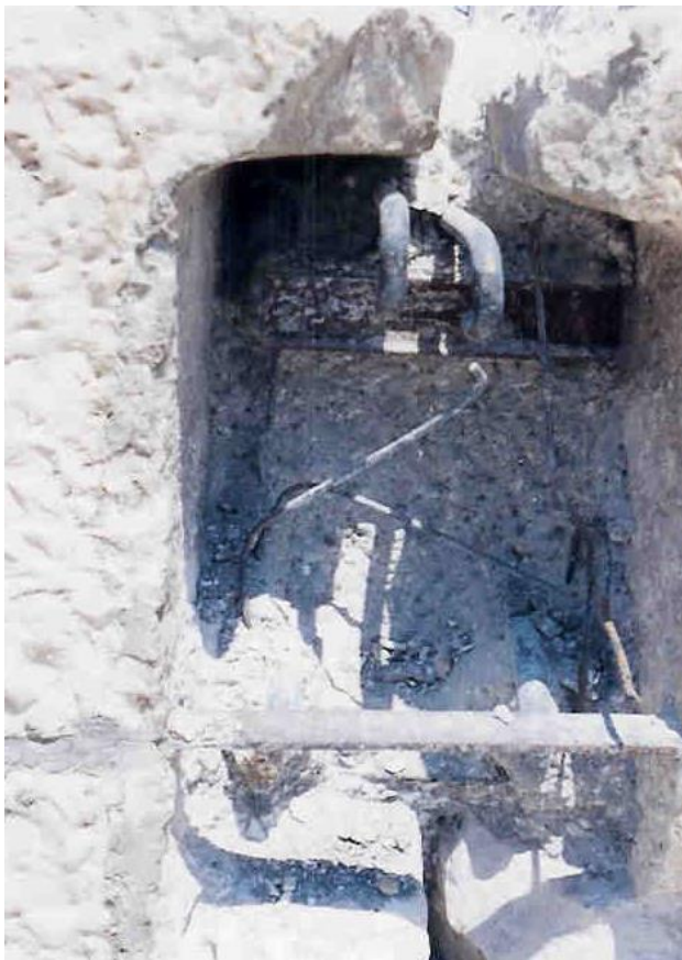
Figure 33b: reinforcement of a member with concrete and iron from past restorations (source: Vacharopoulou, personal photographs -- 2002).
