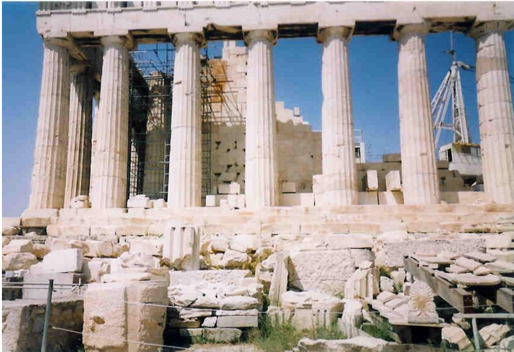
Figure 56b: close view of the south side of the Parthenon during anastylosis (source: Vacharopoulou -- personal photographs, 2002).
