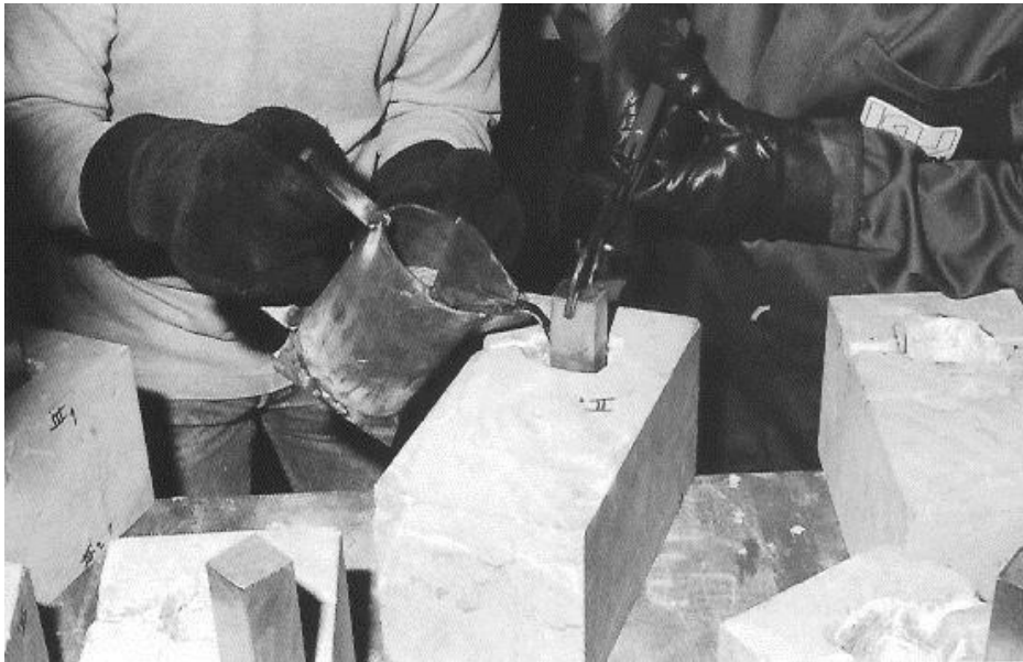
Figure 211a: preparation of the dowels according to the ancient technique by pouring the molten lead around the iron dowel (source: Ercan et al. 1997, 431).
