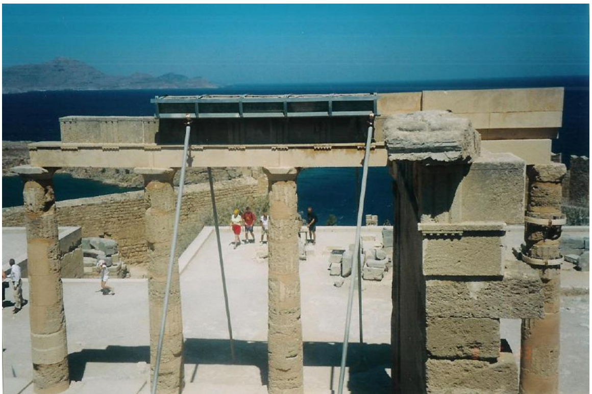
Figure 127: view of the restored transverse colonnade and the restored east wall of the Stoa (source: Vacharopoulou -- personal photographs, 2003).
