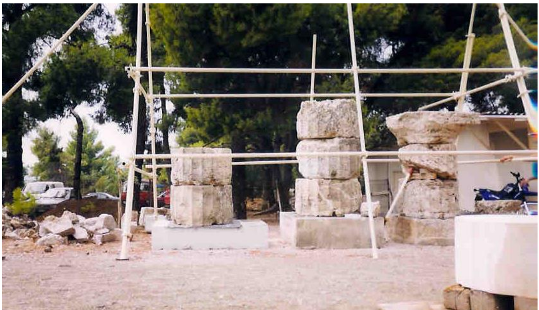
Figure 88: view of restored columns of the Gymnasium Propylon (source: Vacharopoulou -- personal photographs, 2002).
