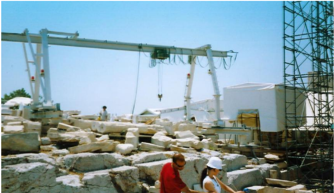
Figure 51a: view of the worksite of the Parthenon (source: Vacharopoulou – personal photographs, 2002).
