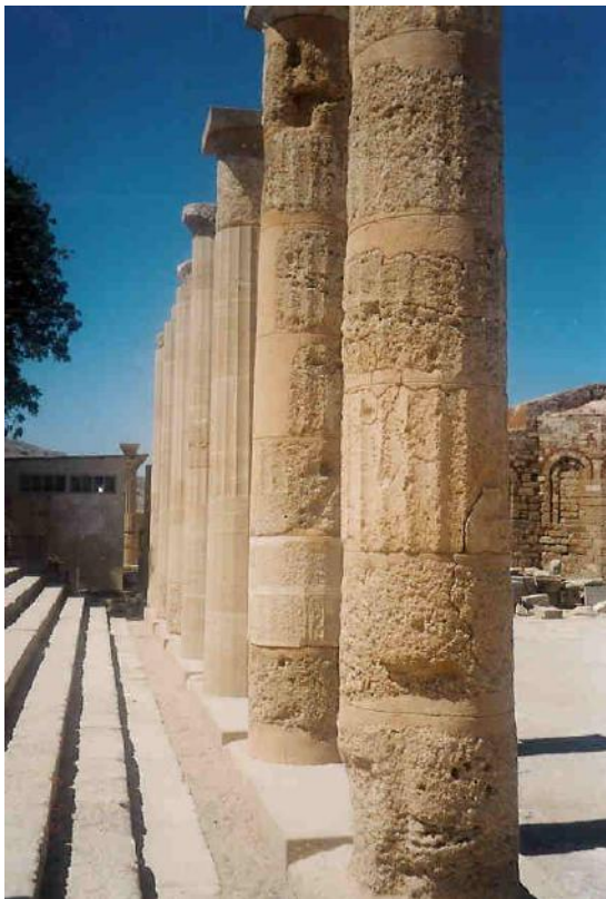
Figure 143b: view of the restored columns of the transverse colonnade of the stoa, indicating the compromise between preservation of form and limited possibility of reuse of original material (source: Vacharopoulou -- personal photographs, 2003).
