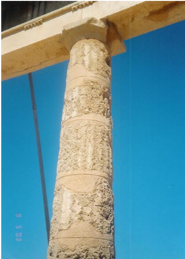
Figure 140a: close view of the column and entablature of the transverse colonnade of the stoa (source: Vacharopoulou -- personal photographs, 2003)
