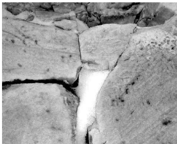
Figure 35b: crack widened by freezing (source: Maurommatis 2003, 20).
