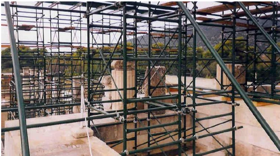
Figure 81b: anastylosis works in the Avaton Stoa with integration of new and original members (source: Vacharopoulou -- personal photographs, 2002).
