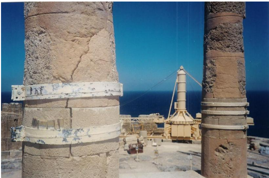
Figure 136c: close view of the columns of the east corner of the stoa that present problems of structural stability (source: Vacharopoulou -- personal photographs, 2003).
