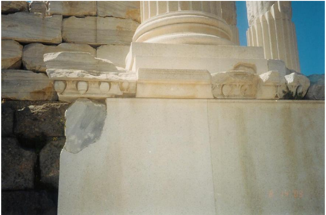
Figure 183c: integration of new and old members, leaving breaks and small defects visible (source: Vacharopoulou -- personal photographs, 2003).
