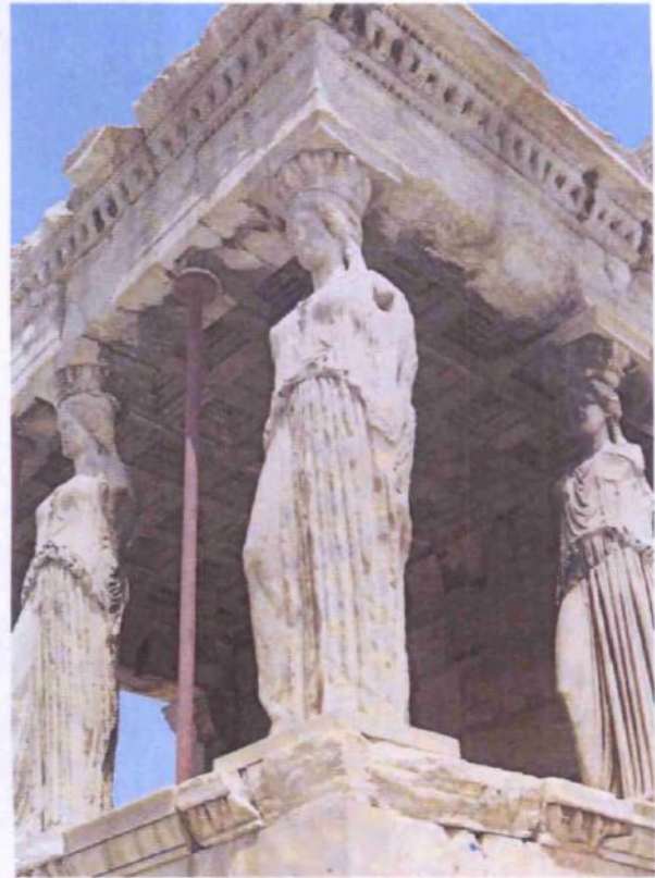
Figure 12b: the southeast corner of the Caryatids porch (1978) before their removal to the Acropolis Museum and the anastylosis (source: Dontas 1979, 69).
