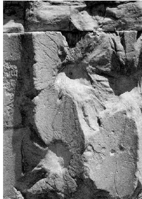
Figure 36b: cracks made by canon-balls and bullets in a column drum (source: Maurommatis 2003, 17)
