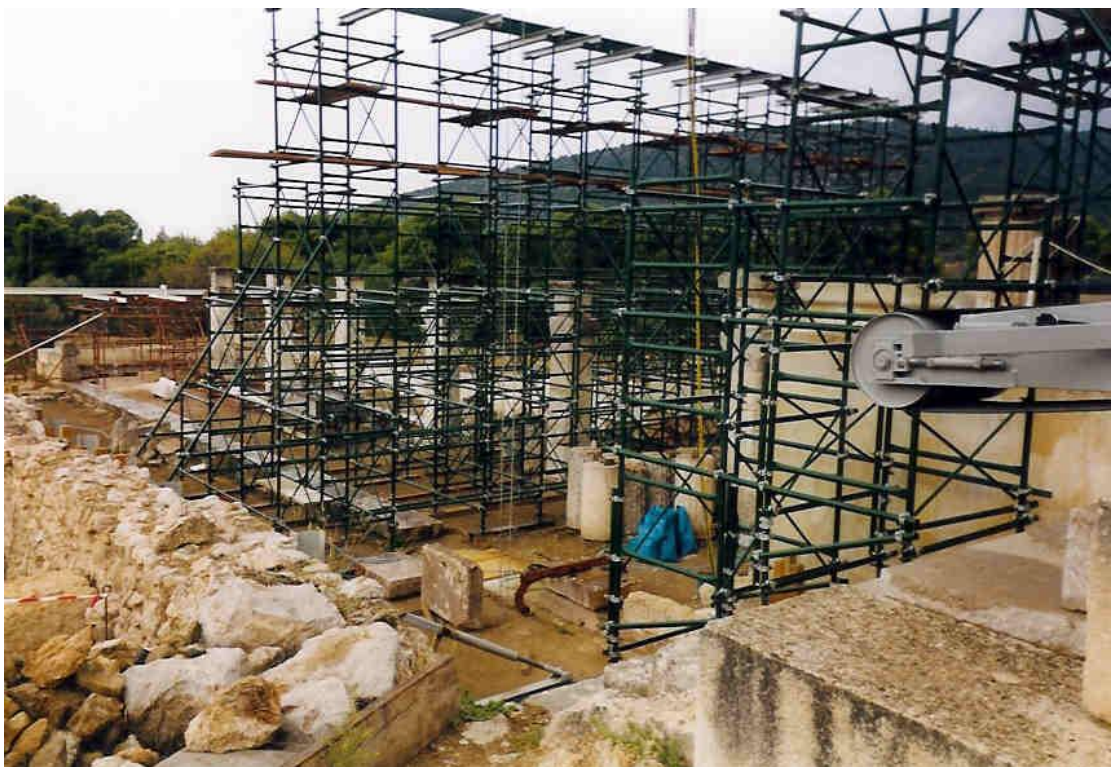
Figure 76d: works in the Avaton Stoa, for consolidating its surviving parts (source: Vacharopoulou -- personal photographs, 2002).
