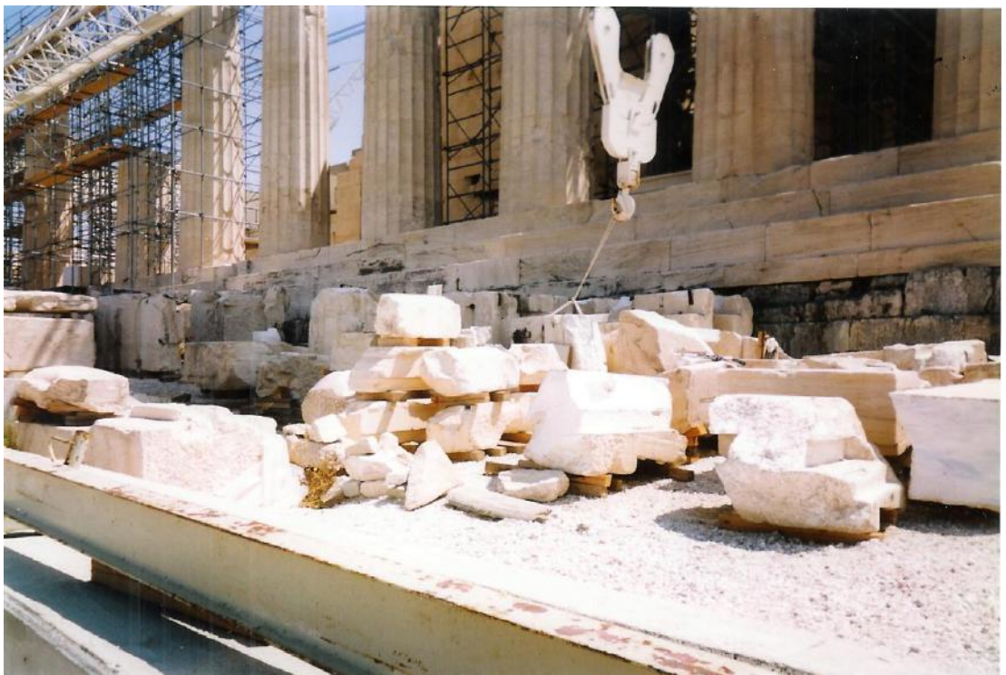
Figure 51b: view of the worksite of the Parthenon (source: Vacharopoulou – personal photographs, 2002).
