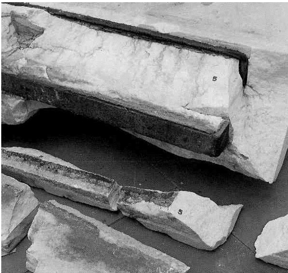
Figure 32b: fracturing of the cornice caused by the swelling of rusted iron clamps introduced in earlier restorations (source: Maurommatis 2003, 18).
