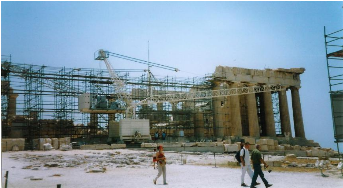
Figure 38: the work-site at the north side of the Parthenon (source: Vacharopoulou -- personal photographs, 2003).
