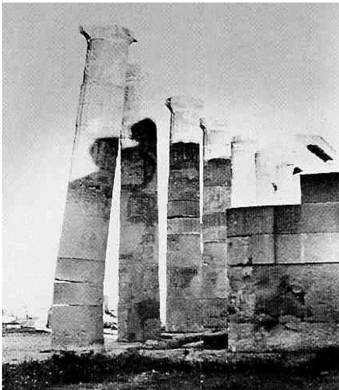
Figure 110: the column of the Stoa ready to fall apart (1972) (source: Eleftheriou 2002i, 46).
