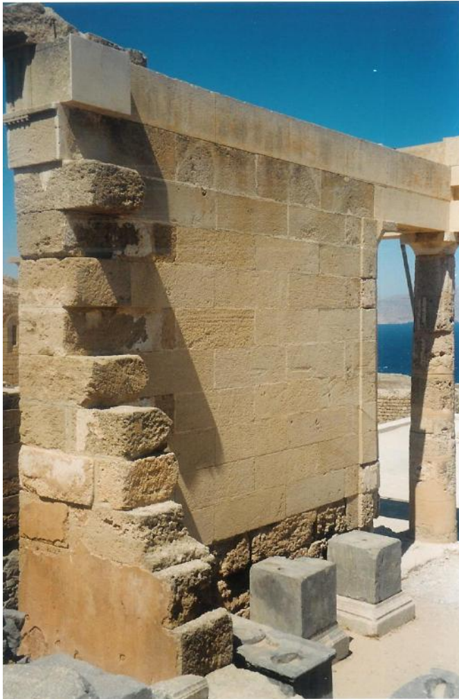
Figure 135c: view of the restored east wall of the stoa (source: Vacharopoulou -- personal photographs, 2003).
