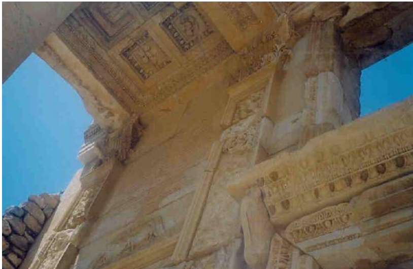
Figure 168b: close view of restored parts of the Library's façade, showing the degree to which ornamentation was copied (source: Vacharopoulou -- personal photographs, 2003).
