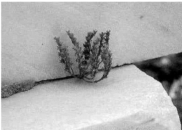
Figure 34b: parasitic plant growth between the column capital and the architrave of the south colonnade of the Parthenon (source: Maurommatis 2003, 20).
