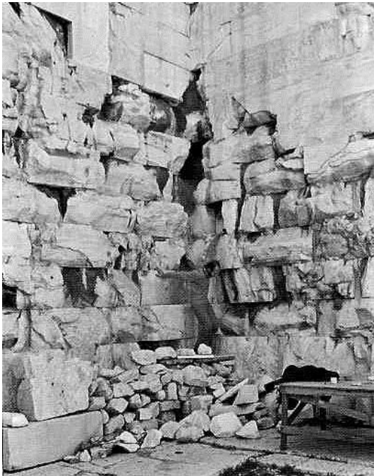
Figure 36a: thermal fracturing of the marble (source: Maurommatis 2003, 16).
