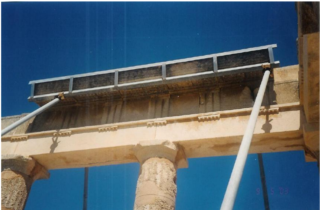
Figure 134a: close view of the restored entablature of the transverse colonnade and the east wall of the stoa, showing the integration of new and original material (source: Vacharopoulou -- personal photographs, 2003).
