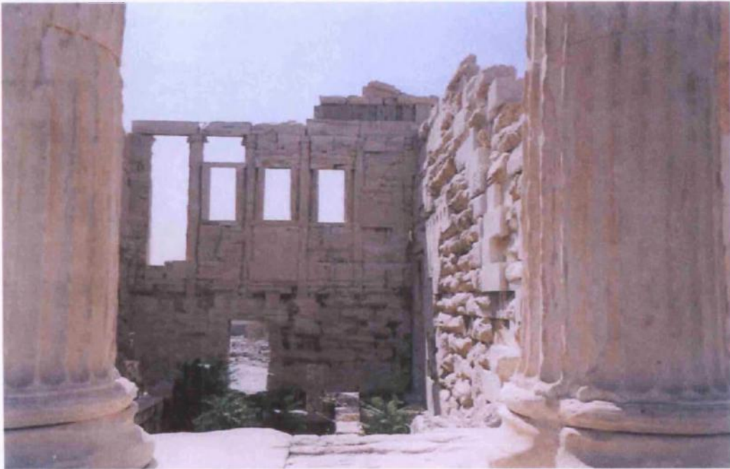
Figure 23: view of the east side and the interior of the Erechtheion, after the anastylosis (source: Vacharopoulou, personal photographs -- 2002).
