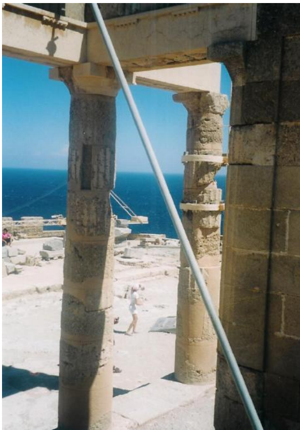
Figure 137c: columns of the transverse colonnade of the stoa that present problems of structural stability (source: Vacharopoulou -- personal photographs, 2003).
