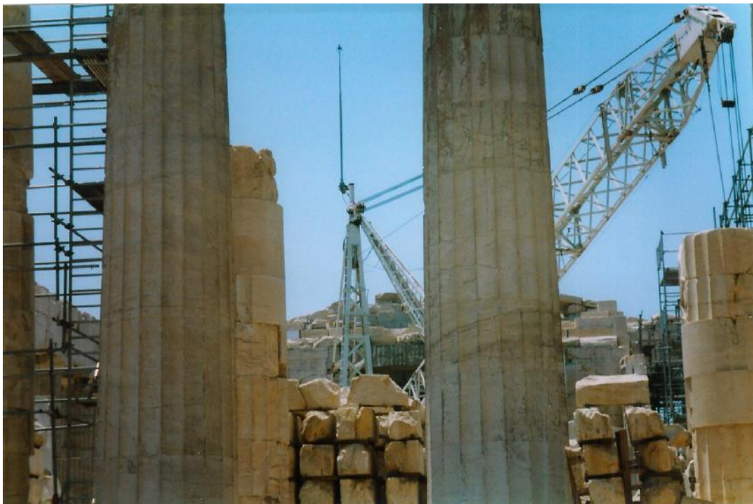
Figure 51d: view of the worksite of the Parthenon (source: Vacharopoulou – personal photographs, 2002).
