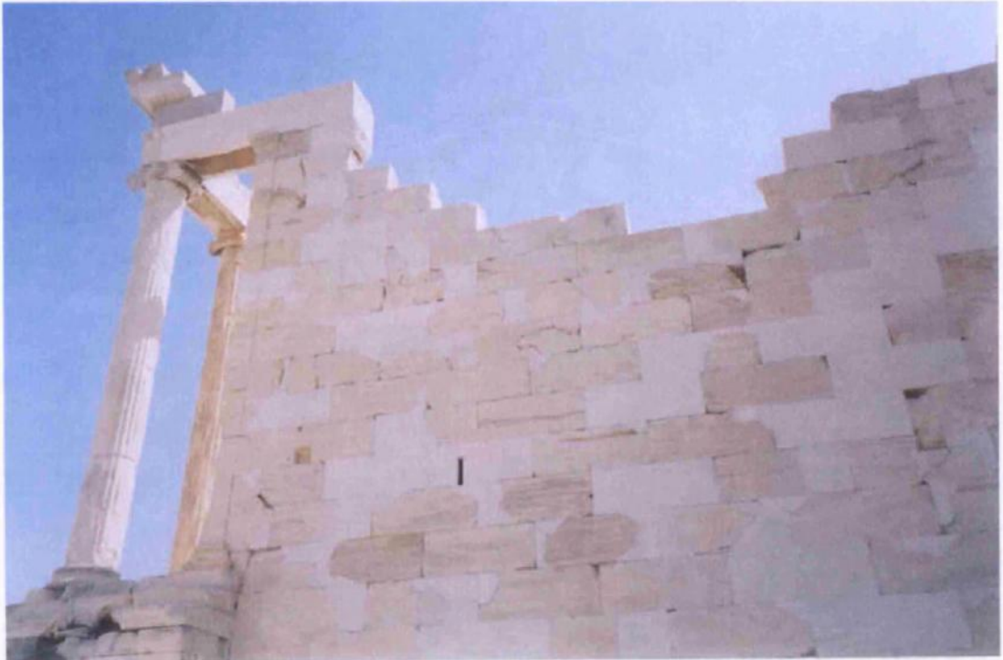
Figure 27a: view of the restored south wall of the Erechtheion, showing the visual contrast between new and old structural members (source: Vacharopoulou, personal photographs -- 2002).
