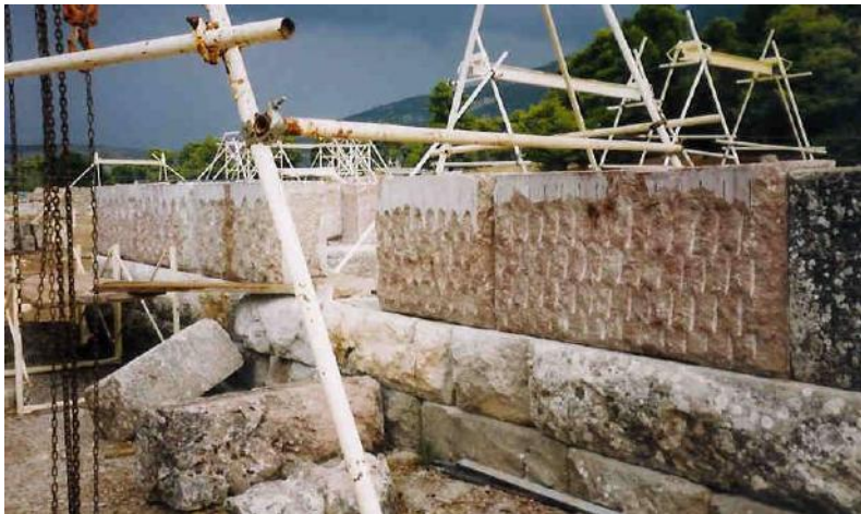
Figure 86b: anastylosis on the Gymnasium Propylon showing how exposed surfaces will be protected by reassembly of old members and integration of new ones (source: Vacharopoulou -- personal photographs, 2002).
