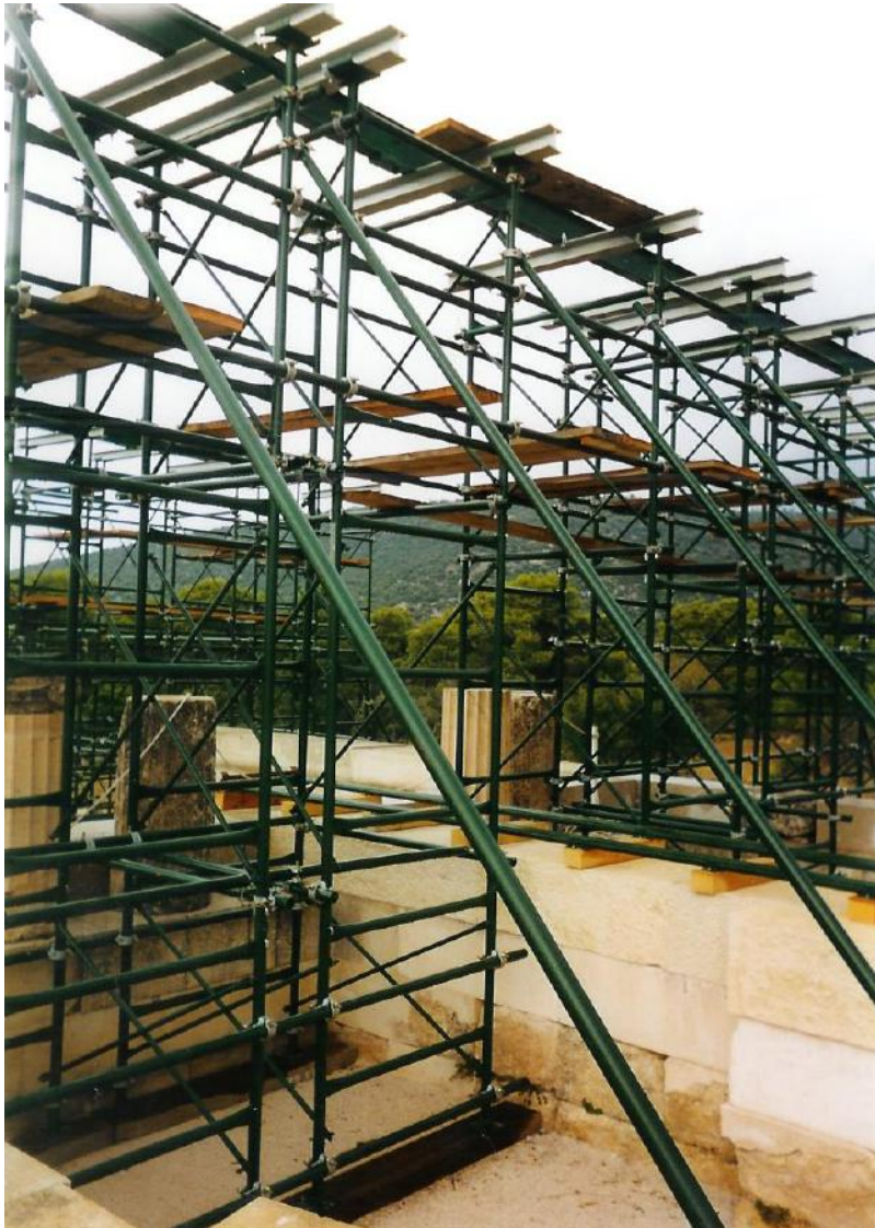
Figure 83: close view of the anastylosis works at the Stoa (source: Vacharopoulou -- personal photographs, 2002).
