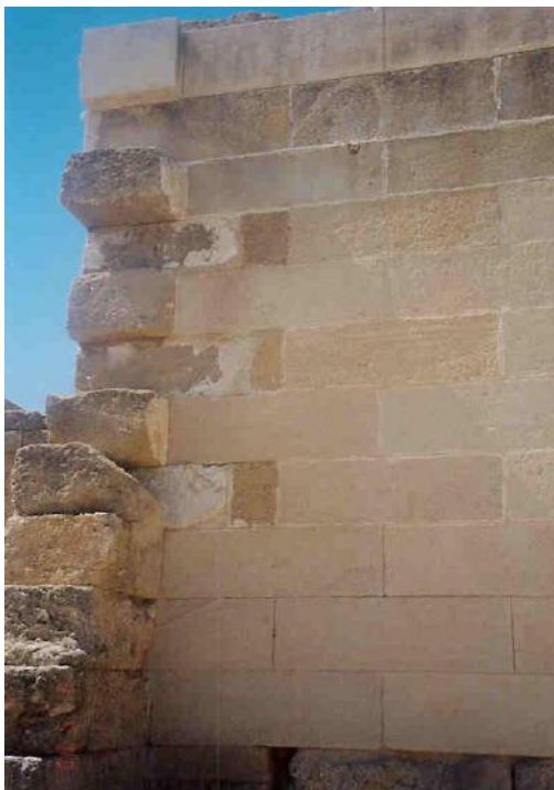
Figure 135d: view of the restored east wall of the stoa (source: Vacharopoulou -- personal photographs, 2003).
