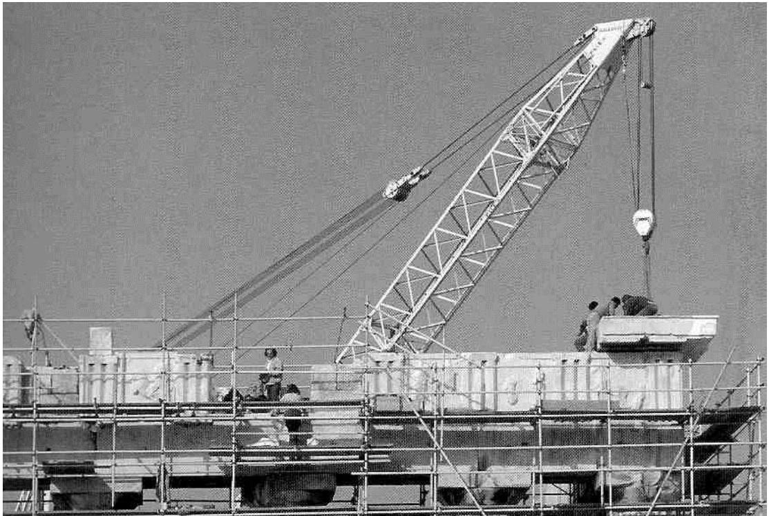
Figure 45a: re-setting of the cornice of the east end of the Parthenon (1990) (source: Maurommatis 2003, 25).
