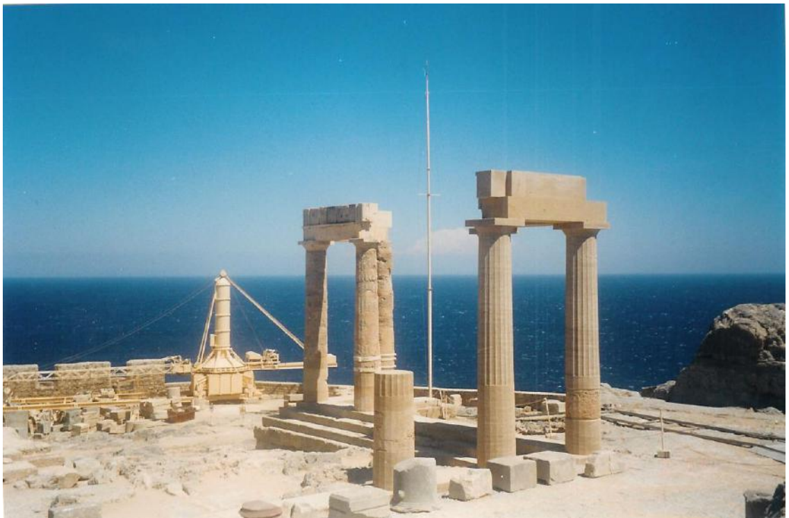
Figure 115b: the work-site near the stoa, inside the archaeological site (source: Vacharopoulou -- personal photographs, 2003).
