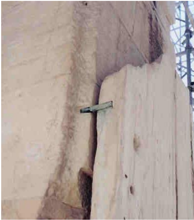
Figure 33a: rusted iron clamp introduced in earlier restorations (source: Vacharopoulou, personal photographs -- 2002).
