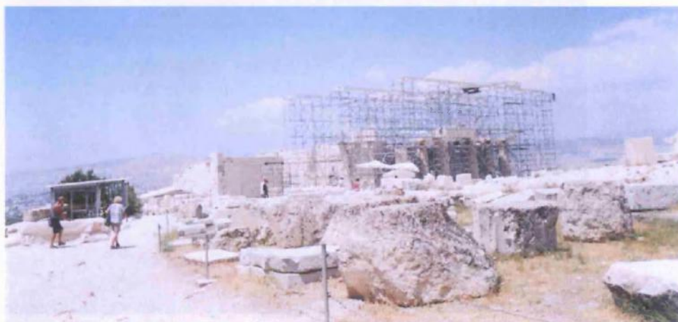
Figure 7c: View of the Propylaea from the south-east during anastylosis works (source: Vacharopoulou, personal photographs – 2002).
