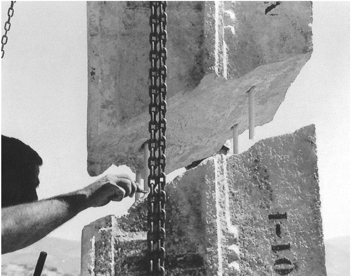
Figure 212: field application of the joining of an architrave block (source: Ercan et al. 1997, 436).
