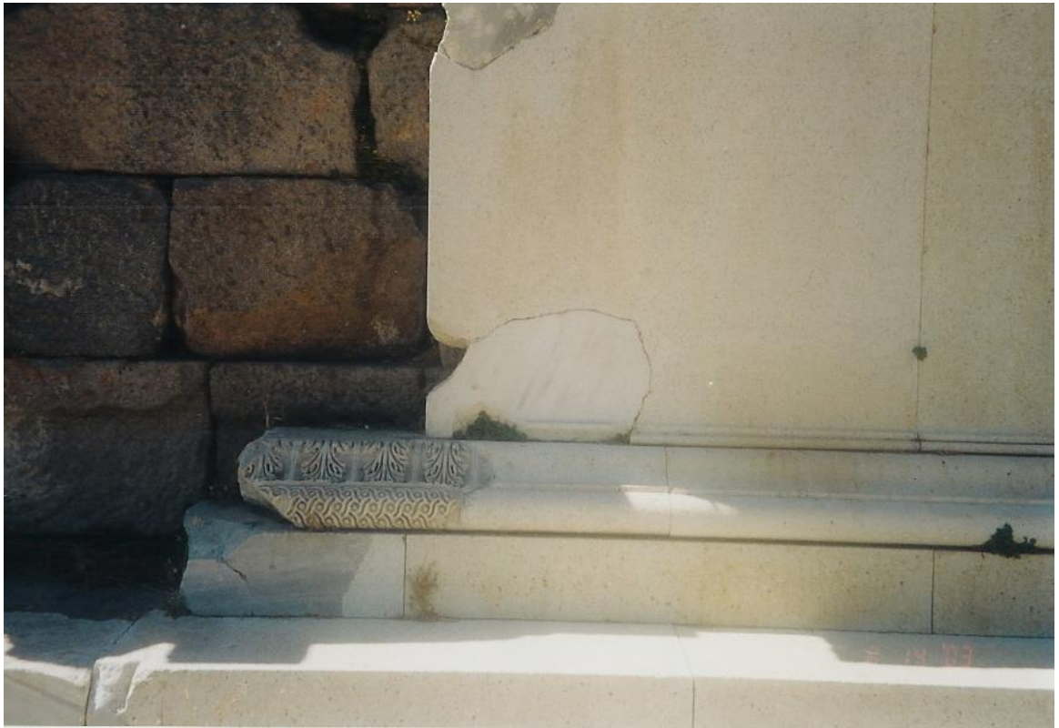
Figure 183a: integration of new and old members, leaving breaks and small defects visible (source: Vacharopoulou -- personal photographs, 2003).
