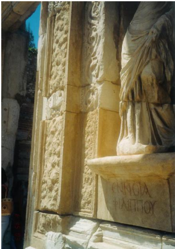
Figure 165b: close view of the restored façade of the Library, showing the replacement of missing members and their differentiation from the original material (source: Vacharopoulou -- personal photographs, 2003).
