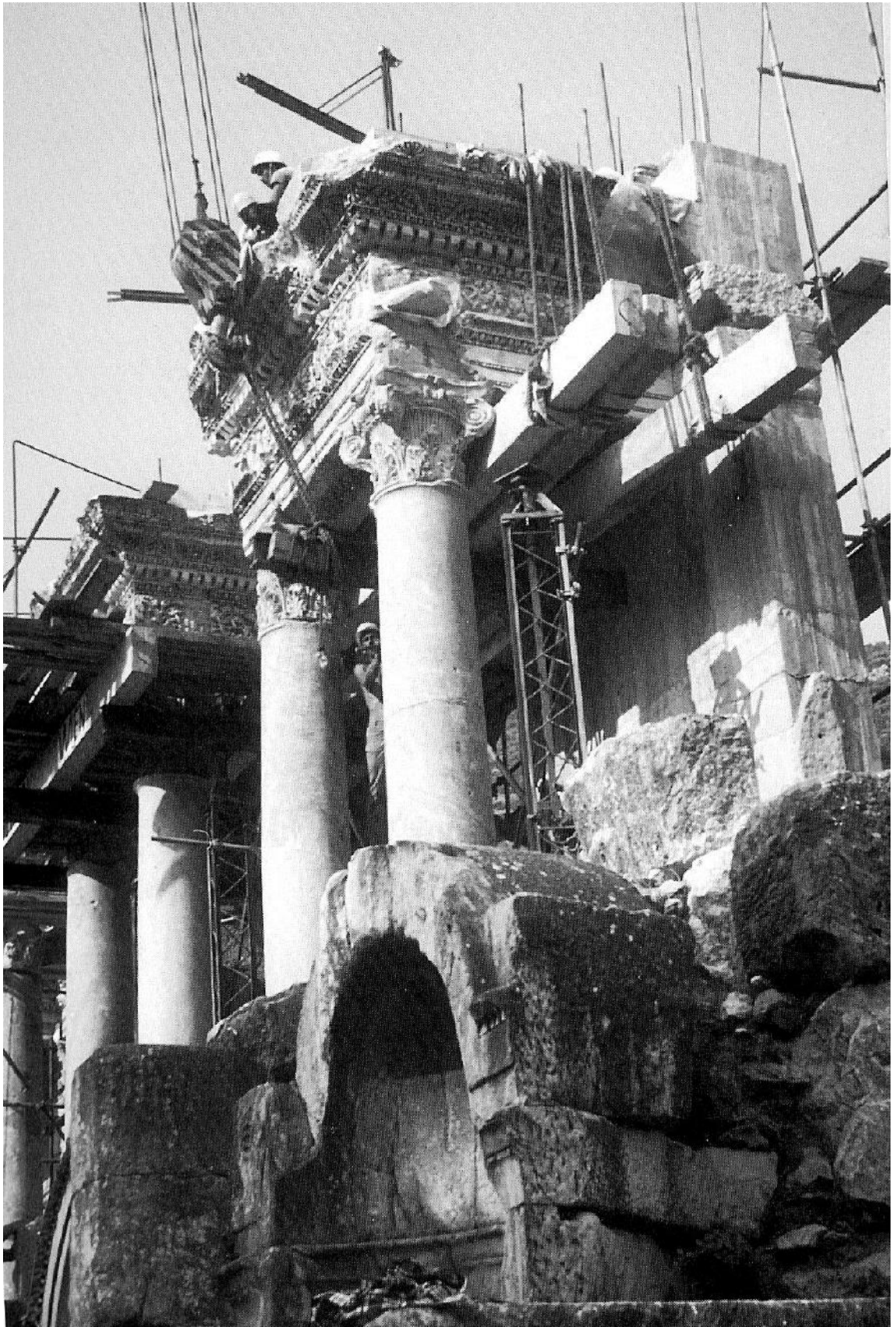
Figure 162: removing the beams supporting the ground floor architrave of the Celsus Library (1975) (source: Wiplinger and Wlach 1996, 123).
