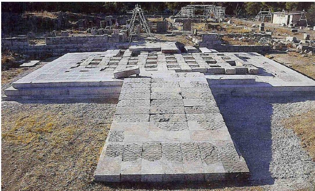
Figure 90: the Gymnasium Propylon after restoration of the crepis up to the second stair (source: Kyriaki 1999, 38).
