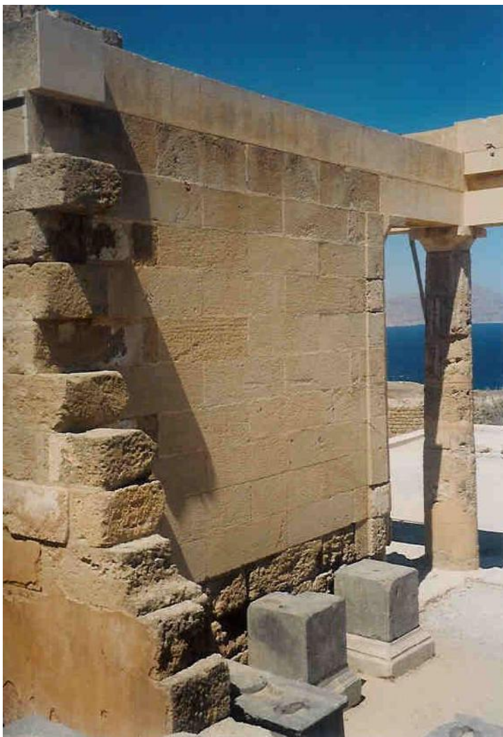
Figure 123b: close view of the restored east wall of the stoa (source: Vacharopoulou -- personal photographs, 2003).
