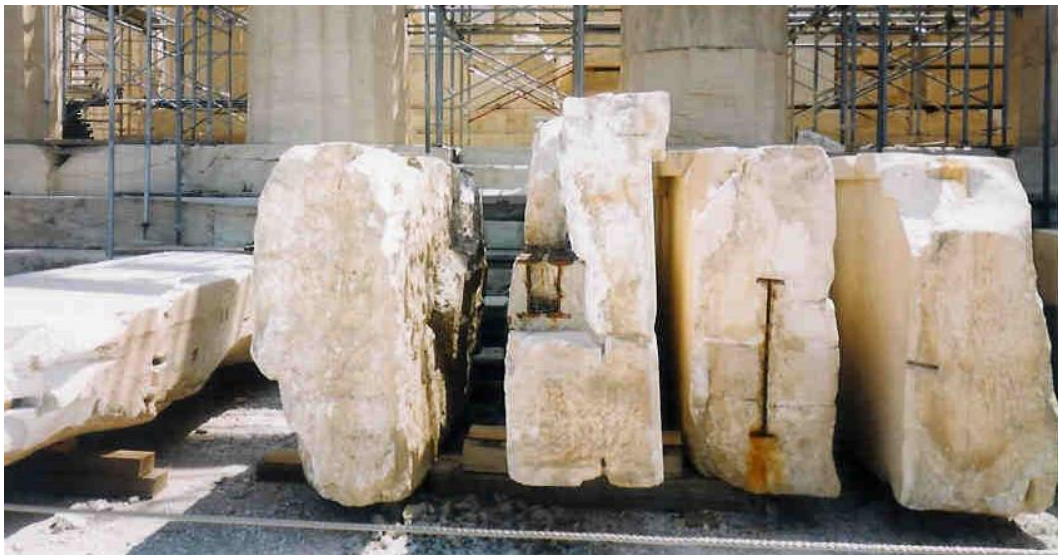
Figure 64a: close view of members used in past restorations and suffering erosion damages (source: Vacharopoulou -- personal photographs, 2002).
