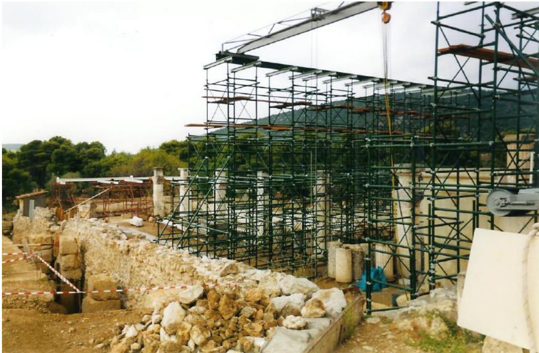
Figure 76c: works in the Avaton Stoa, for consolidating its surviving parts (source: Vacharopoulou -- personal photographs, 2002).
