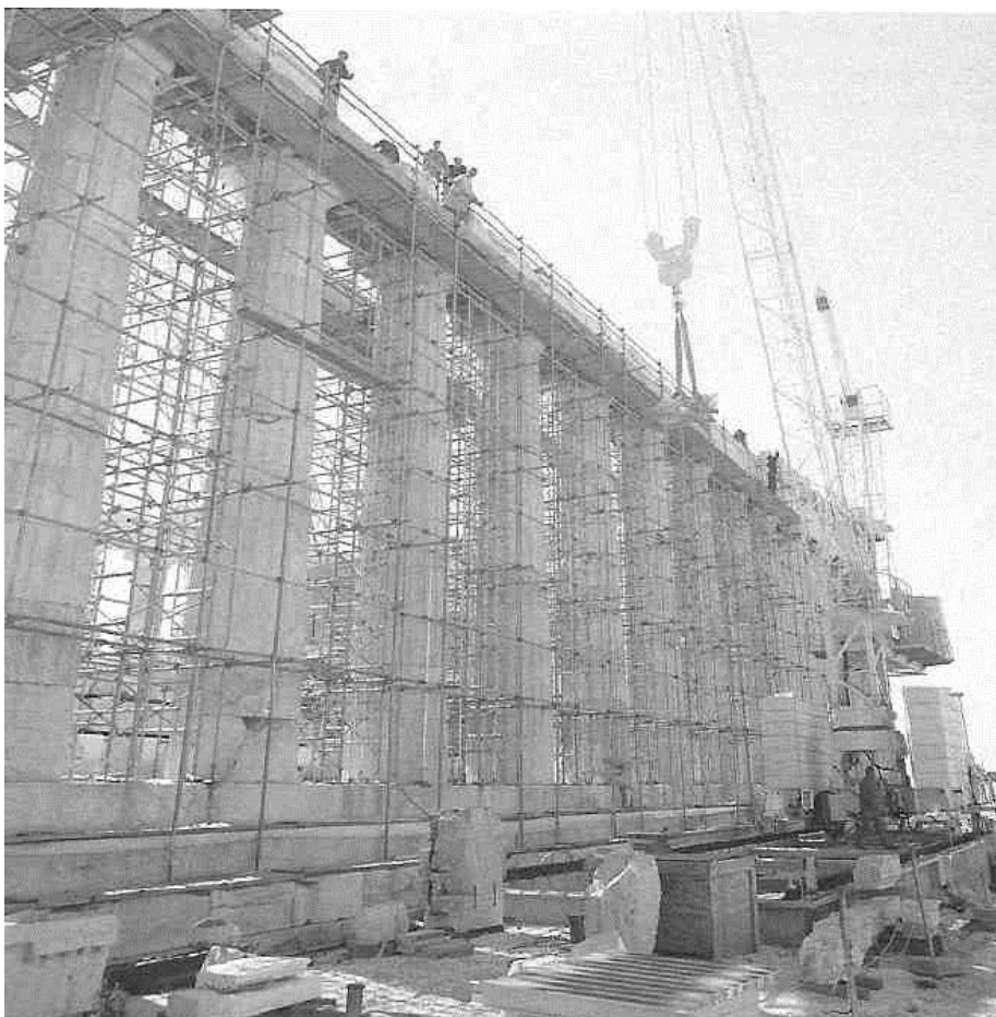
Figure 39a: dismantling the cornices of the Parthenon north colonnade (photo by Bouras, 2001) (source: SRAM 2002, 14).
