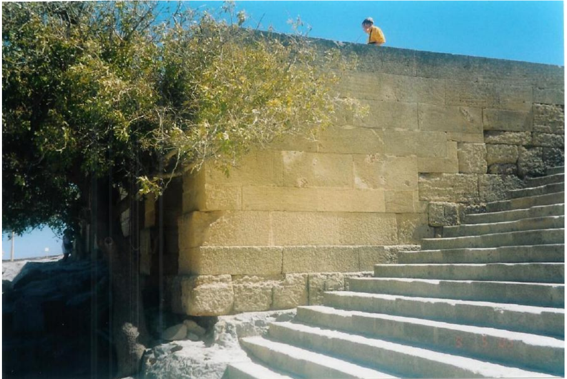
Figure 145a: View of the left vault, inside which structural members not used in the anastylosis are exhibited (source: Vacharopoulou -- personal photographs, 2003).
