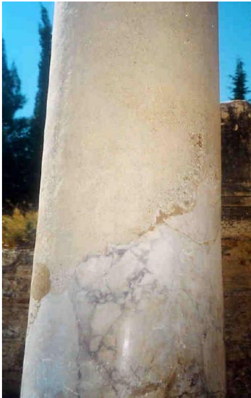
Figure 169a: close view of a restored column showing how harmonious but distinguishable integration of new material was achieved (source: Vacharopoulou -- personal photographs, 2003).
