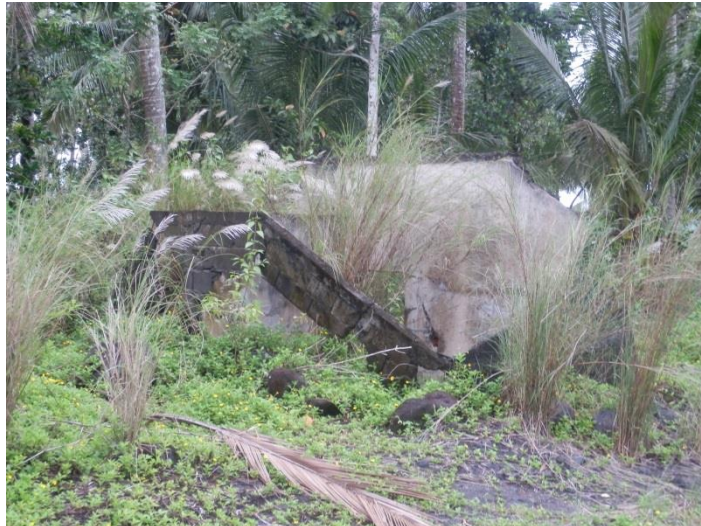
Figure 7.9 The ruins of a concrete home in Tandarora destroyed by lahars during Reming (October 2012). Source: author's own
