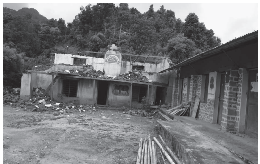
Photo 4 : Dhungagadhe Lower Secondary School 5 of all 7 classroom, teachers room buildings were broken. Only 3 rooms built by Japanese Aid in 1990's (left) are remained but need repairing for use. (August 2015)
