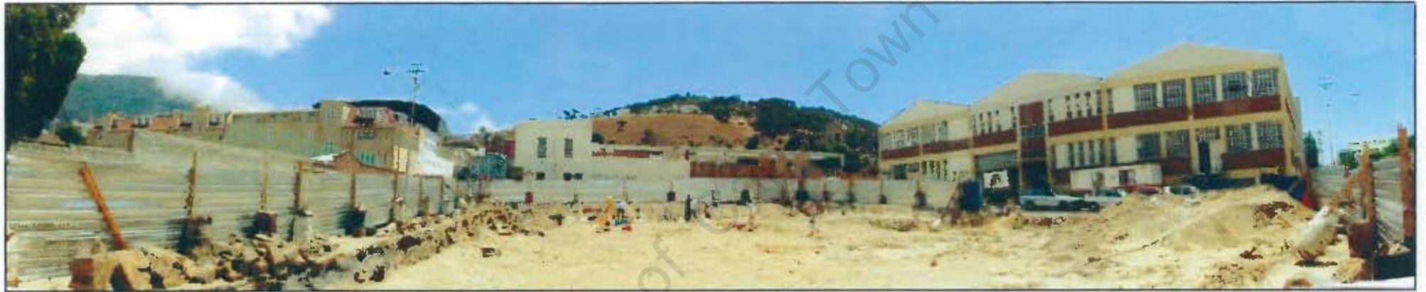
6. Panorama of the site bounded by Prestwich, Alfred, Napier and West Streets, 2003 (Photograph: A. Malan).
