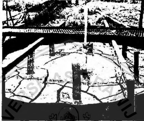
Figure 13: Field trial using electrokinetic prefabricated vertical drains to further dewater thickened mine tailings. The cathode is situated in the centre, surrounded by anodes
