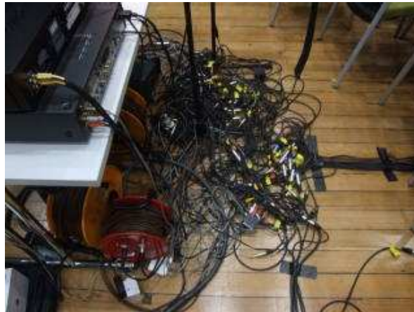
Figure 3. Tangle of cables typical in sound spatialisation setups.
