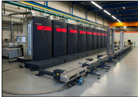
Figure 2-18: Hauzer example of in-line Magnetron sputtering
