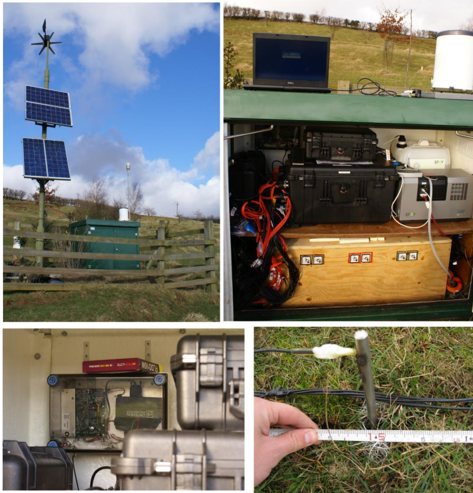
Figure 4.8 a.) (top left) ALERT System installed at Hollin Hill; green secure housing contains monitoring system, batteries and communication modem. To the west of the instrumentation housing is a pole with attached solar panels and wind turbine. b.) (top right) Inside the system housing; two black boxes are the ALERT system, wooden box positioned on the housing floor contains two batteries and the silver box to the right of the housing is a methanol fuel cell (installed ~October 2012). c.) (bottom left) Communication modem and SIM card for uploading data acquisition schedules and downloading survey results. d.) Stainless steel electrode with multicore cable attached before being inserted 0.1 m into the subsurface. Note, accurate electrode positioning by tape measure and later RTK-GPS location measurement.
