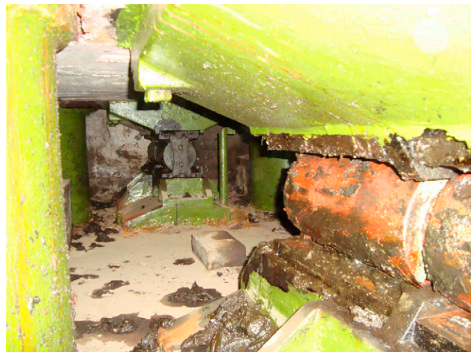
Fig. 3. Roller bearings supporting a bridge pier (image courtesy of Dr. Peter Bennett, taken September 22, 2009)
