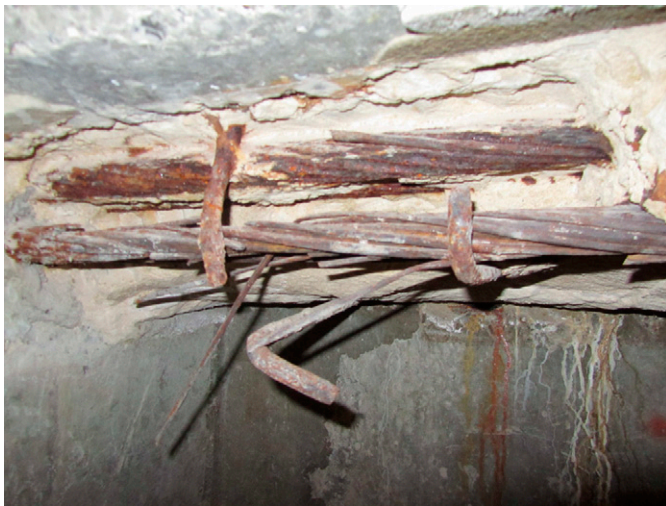
Fig. 2. Corrosion of prestressing tendons (image by authors, taken May 14, 2012)
